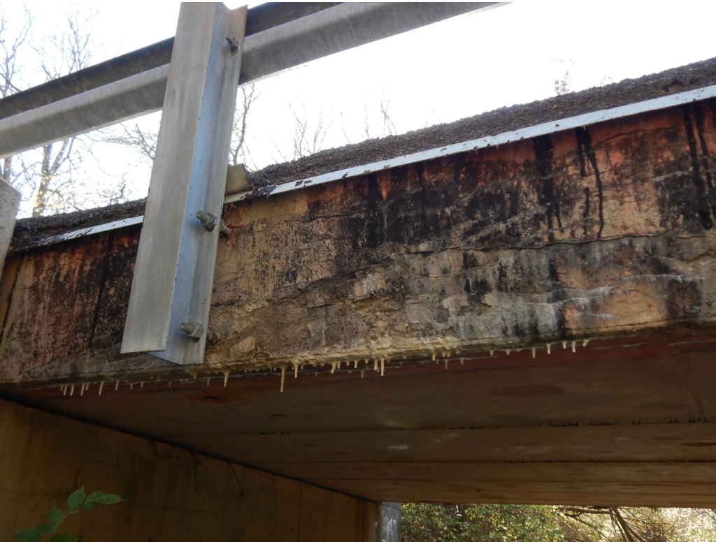
In addition to the right fascia beam, longitudinal cracking, delamination, and efflorescence can be seen along the whole length of the left fascia beam.
