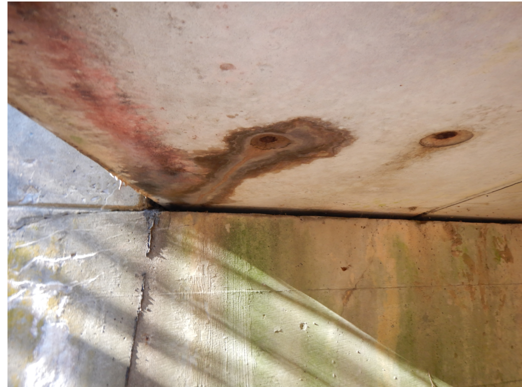
Moisture buildup in the voids of the fascia beams is evident by the wetness and staining around the weep holes.
