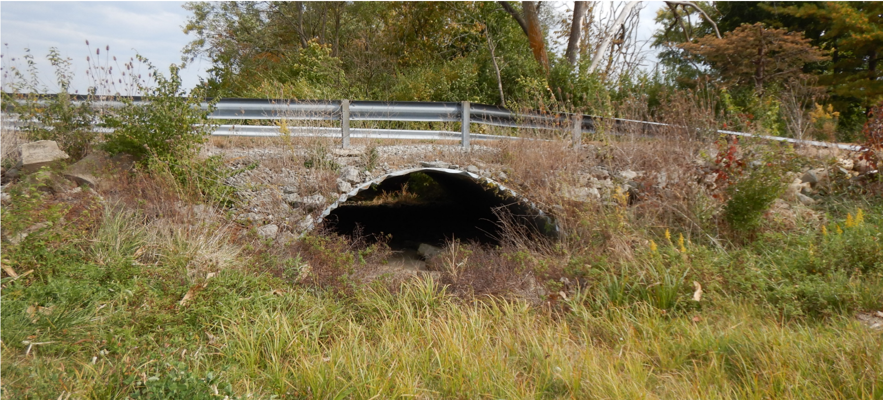
Profile view of the bridge as seen from the West looking East
