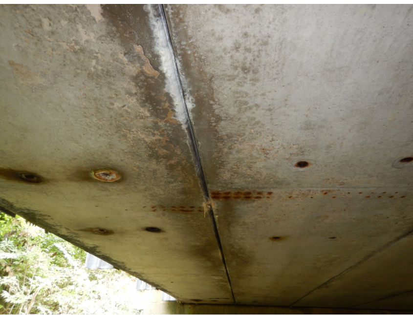
West Exterior Beam Efflorescence
