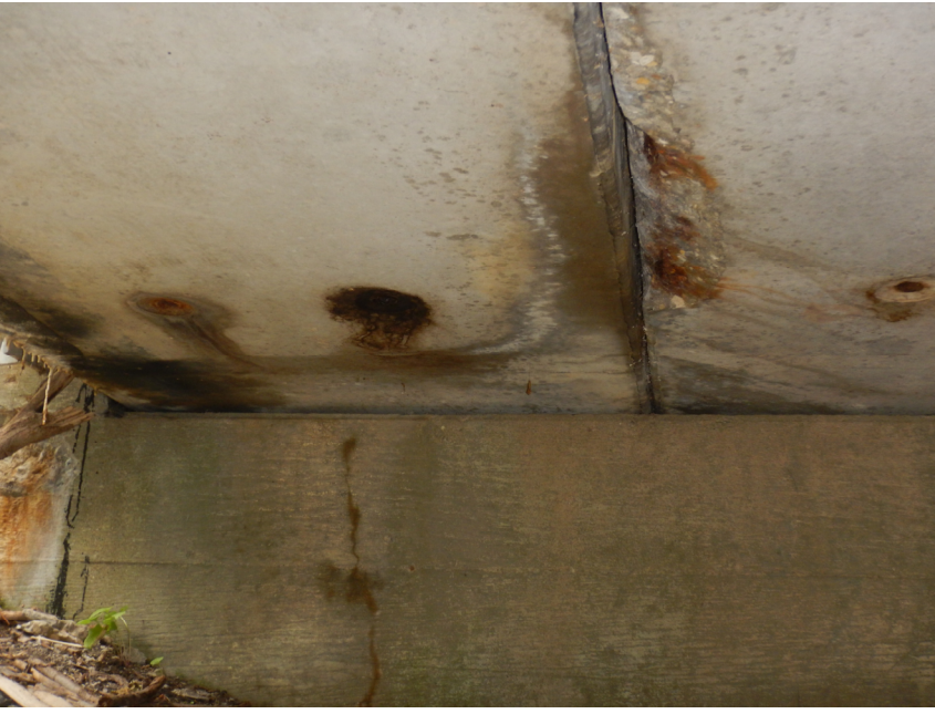
Interior Beam Spall
