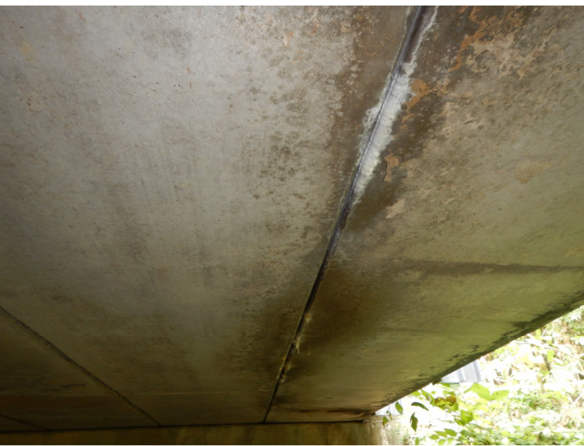
East Exterior Beam Efflorescence
