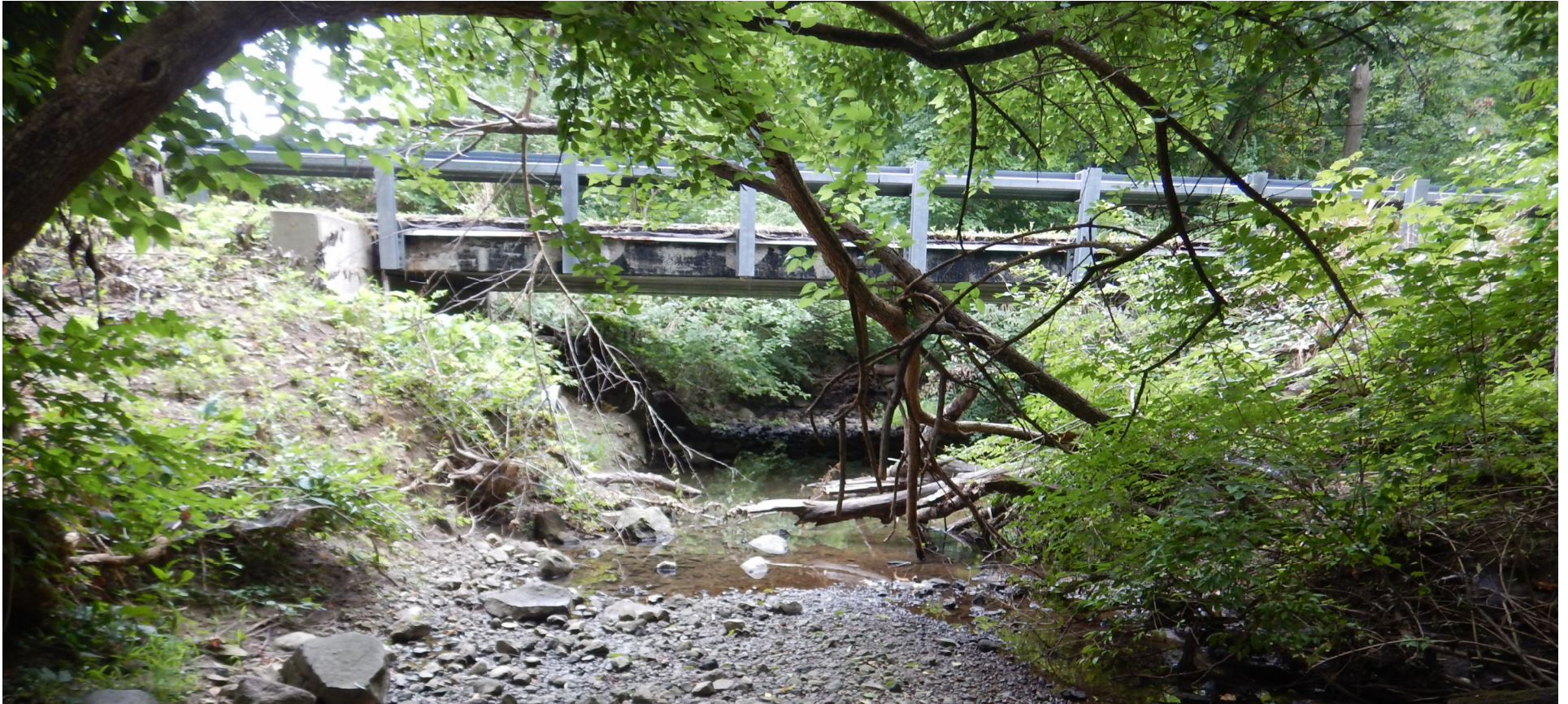
Profile View of the Wellbaum Road Bridge over the Razor Run as seen from the West Looking East
