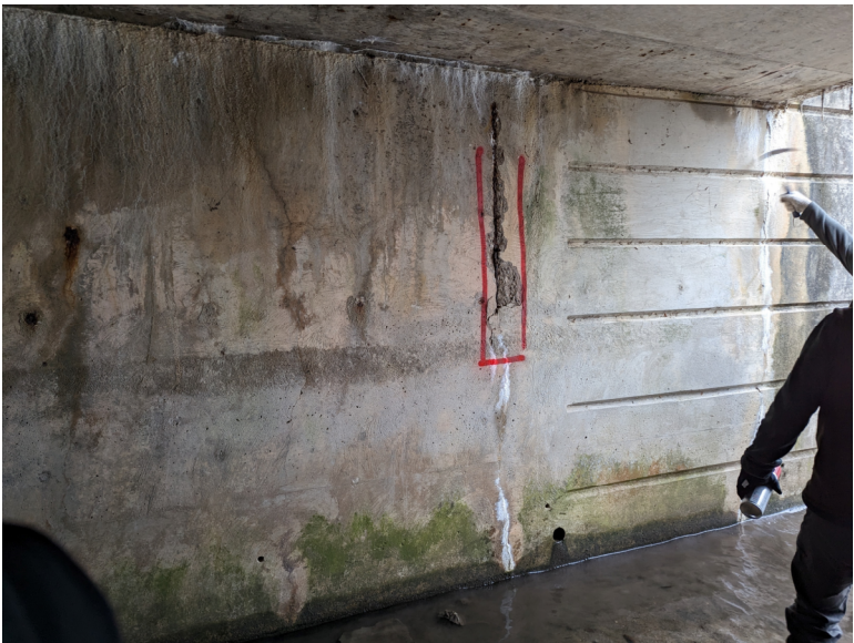
Vertical Crack at Northeast Corner of North Abutment Looking Northeast
