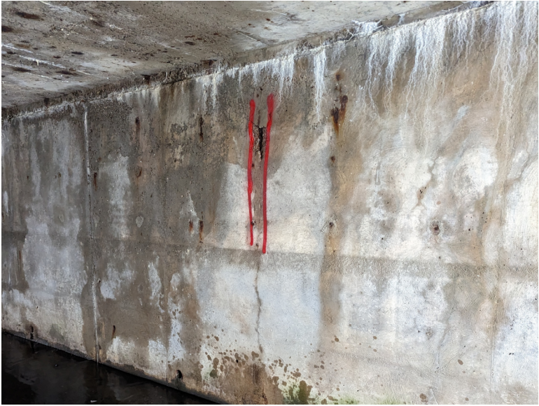
Vertical Crack in East Half of North Abutment Looking Northwest
