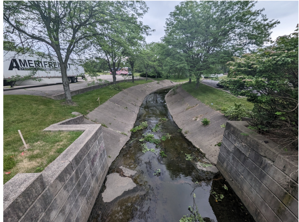
View of the Downstream Channel as seen from the Top of the Bridge Looking East
