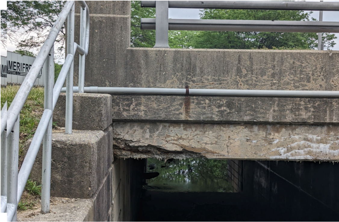
Deterioration of West Exterior Beam at Northwest Corner Looking East
