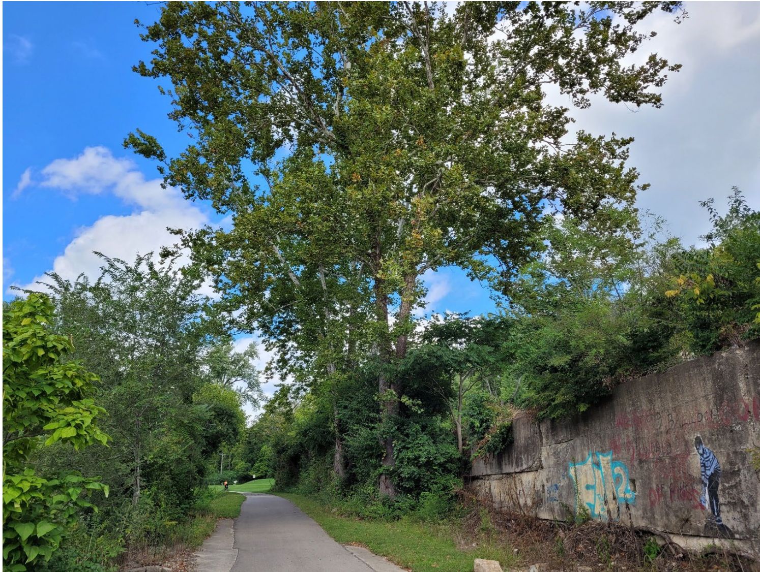
Figure 6: Dayton Cincinnati Pike – North Wall Section Showing Front Face Rotated
