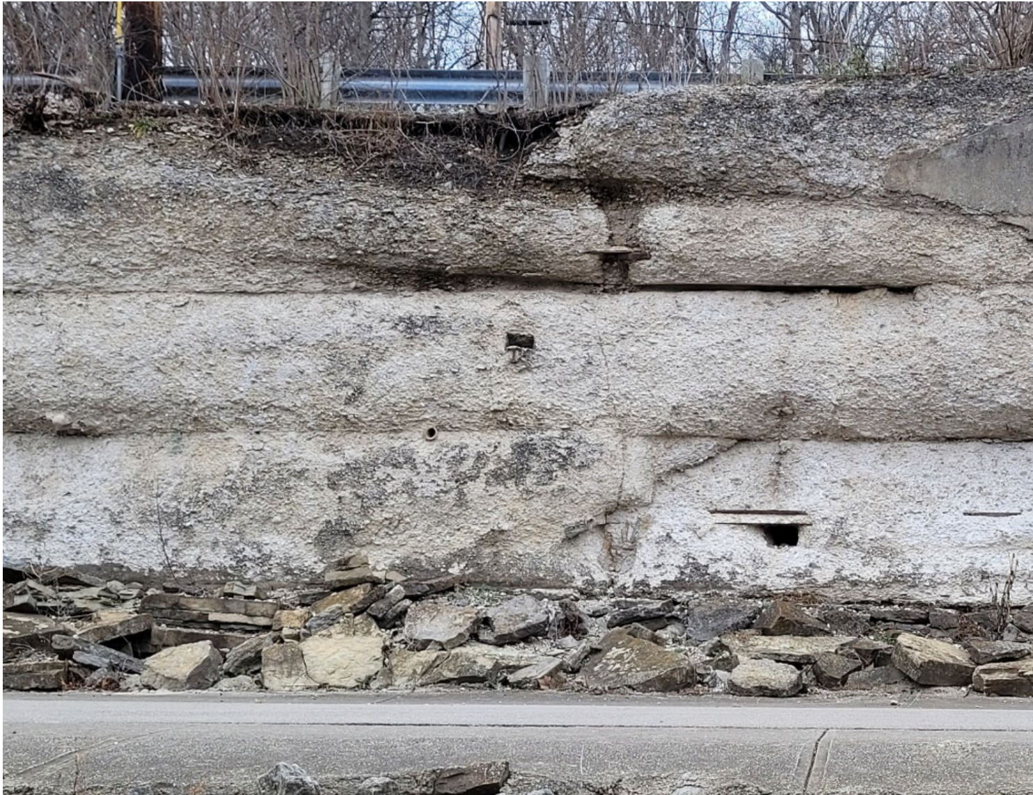
Figure 3: Dayton Cincinnati Pike – Spalled Section at Top of Wall
