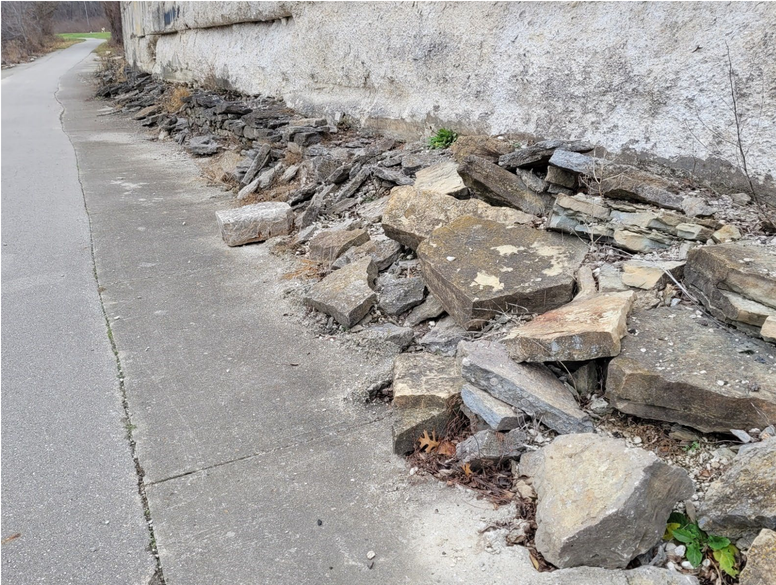
Figure 4: Dayton Cincinnati Pike – Existing Loose Stone Foundation
