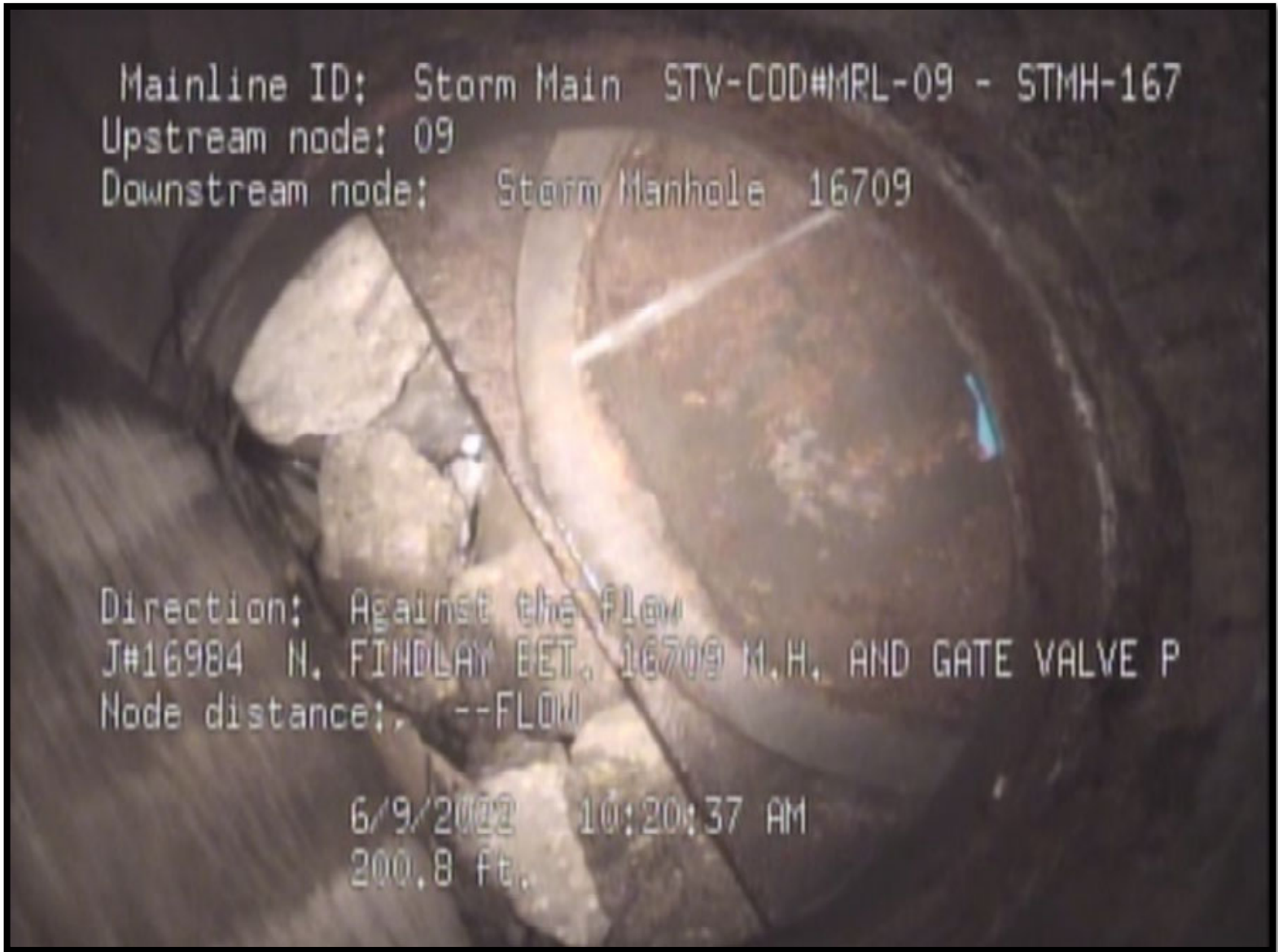
Figure 4 - Jammed sluice gate with rock blockage
