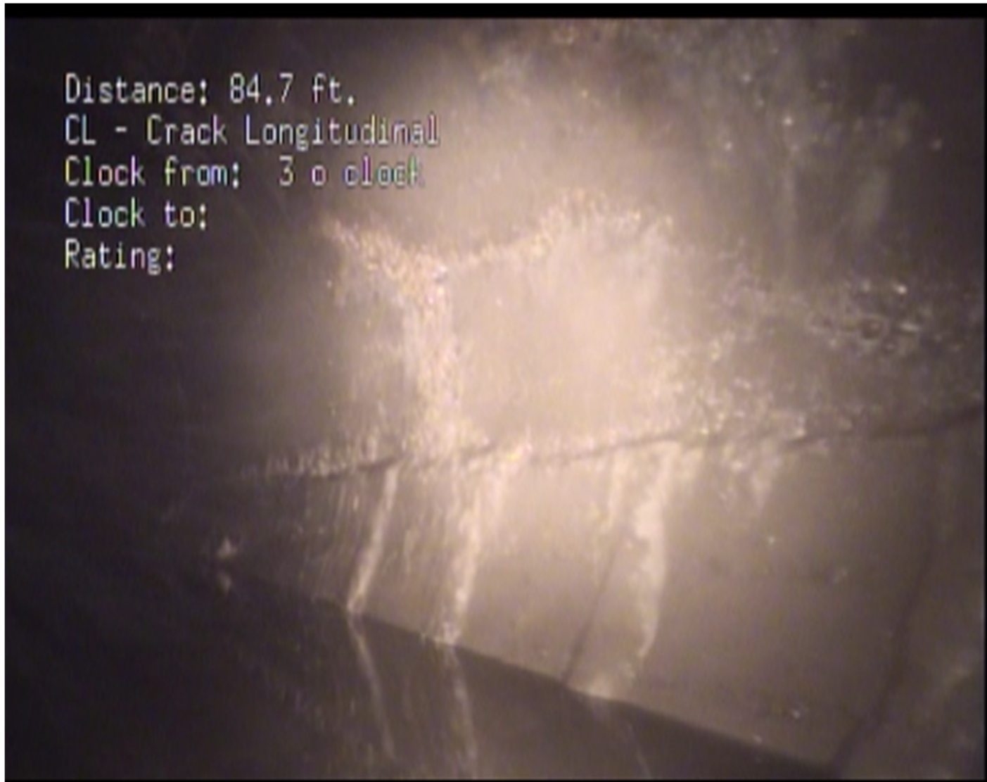
Figure 5 - Crack in 36" pipe between Manholes 30002 and J10ST49491
