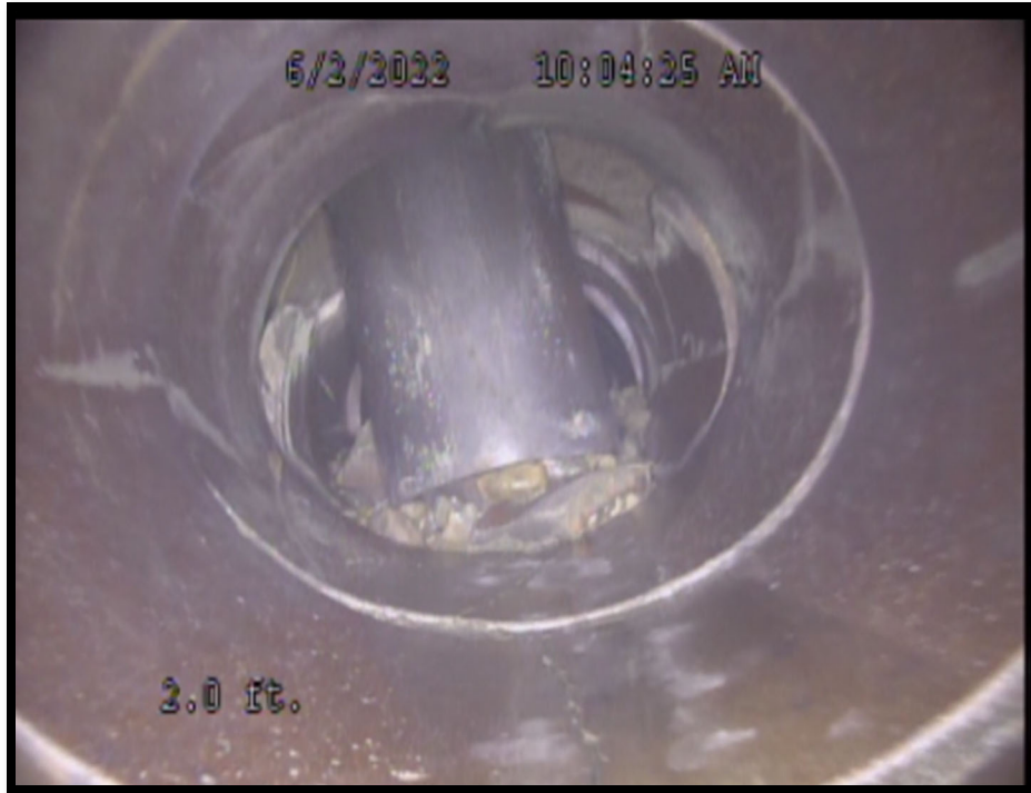
Figure 4- Catch basin that has dropped into the pipe. Storm pipe between Oxford and Lexington Avenues
