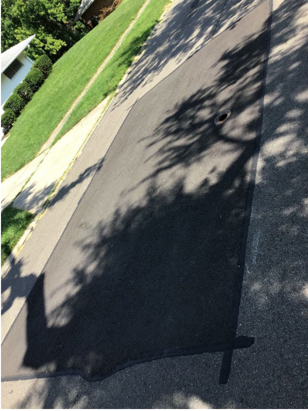
Sunray Rd patch, facing north
