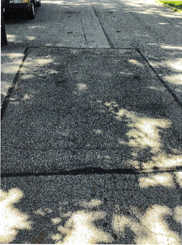
Rio Ln patch, facing west
