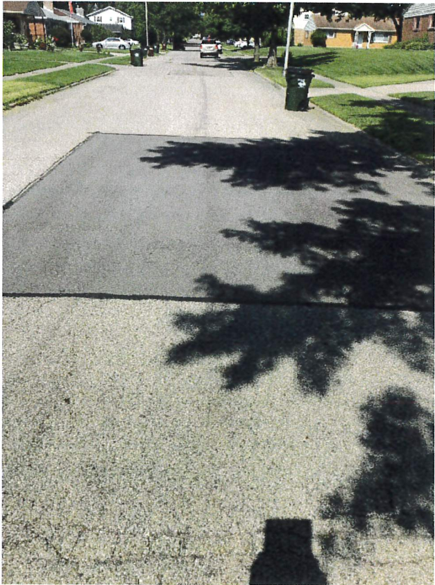
Rio Ln patch, facing west
