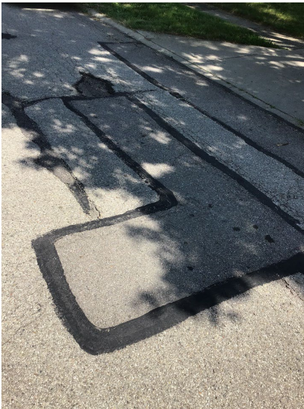
Sunray Rd patches, facing north
