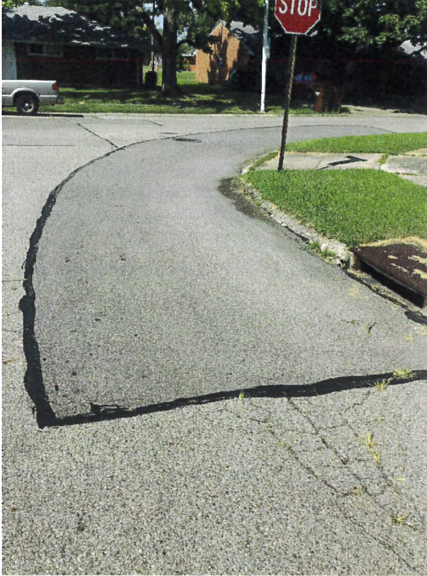
Chee Ct patch, facing southwest
