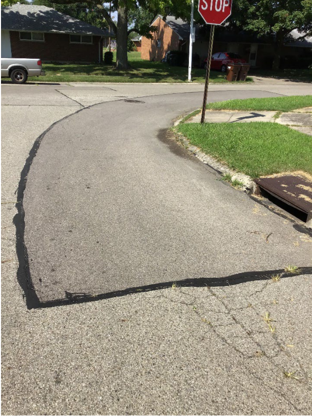
Chee Ct patch, facing southwest
