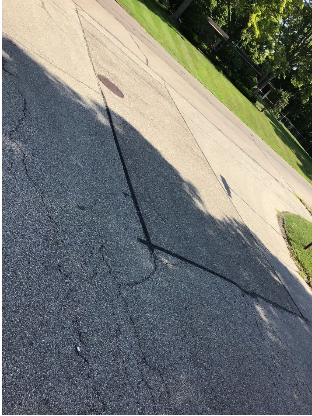
Silbury Lane patch, facing north
