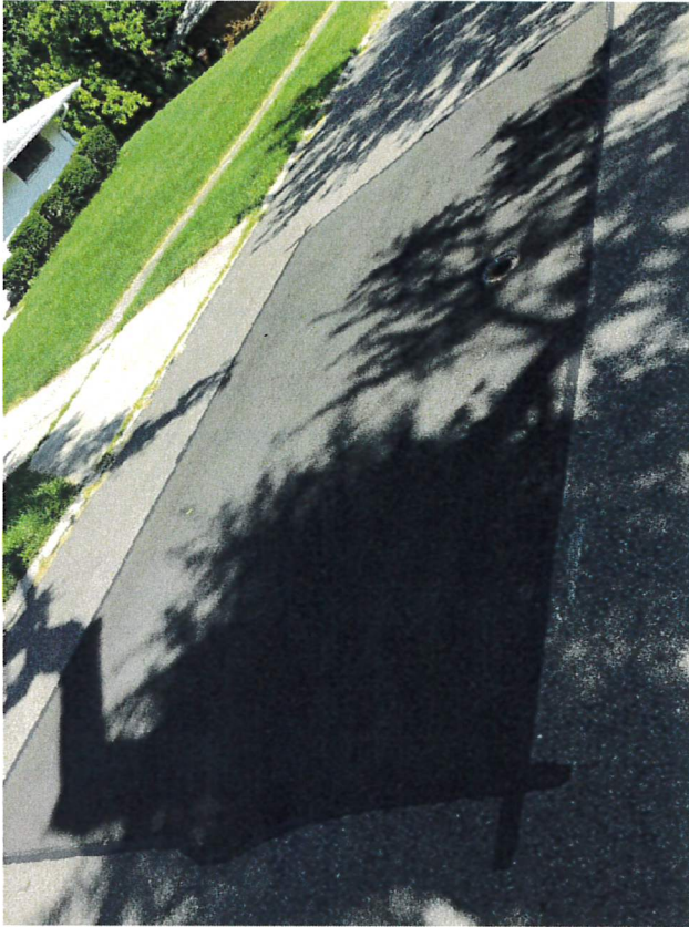
Sunray Rd patch, facing north
