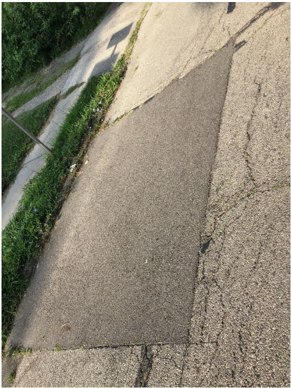
Natchez Ave patch, facing east Natchez, Annapolis, Nevada WMR Project
