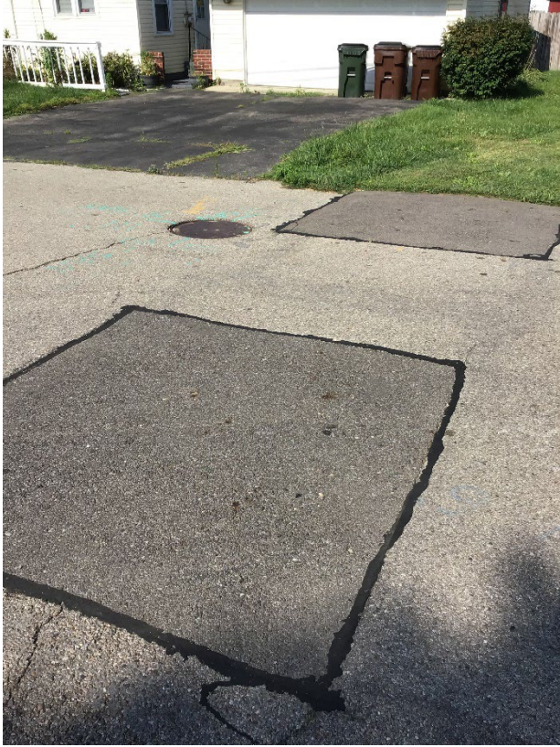
Dexter Ave patches, facing west
