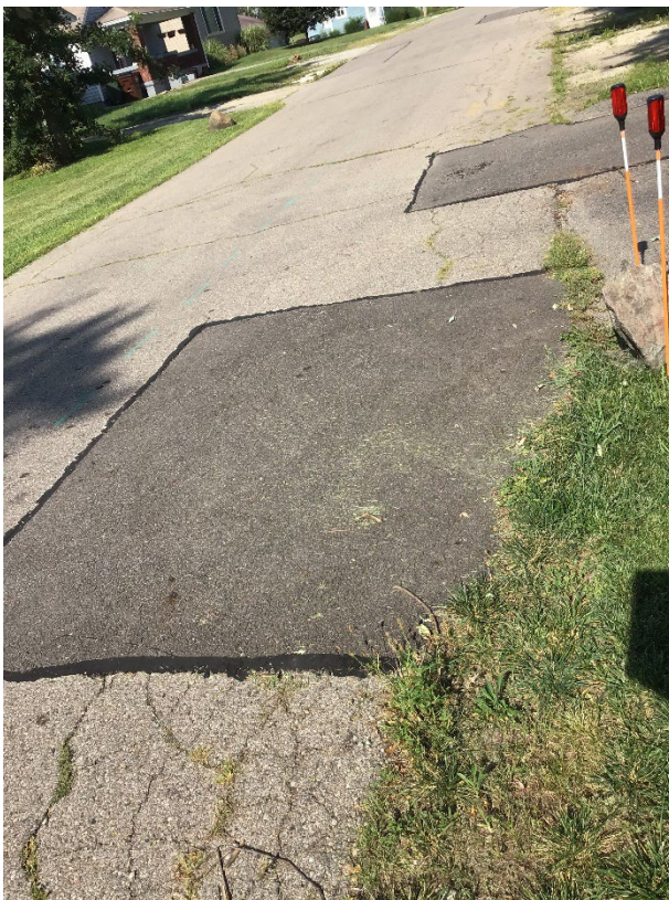
Dexter Ave patches, facing west
