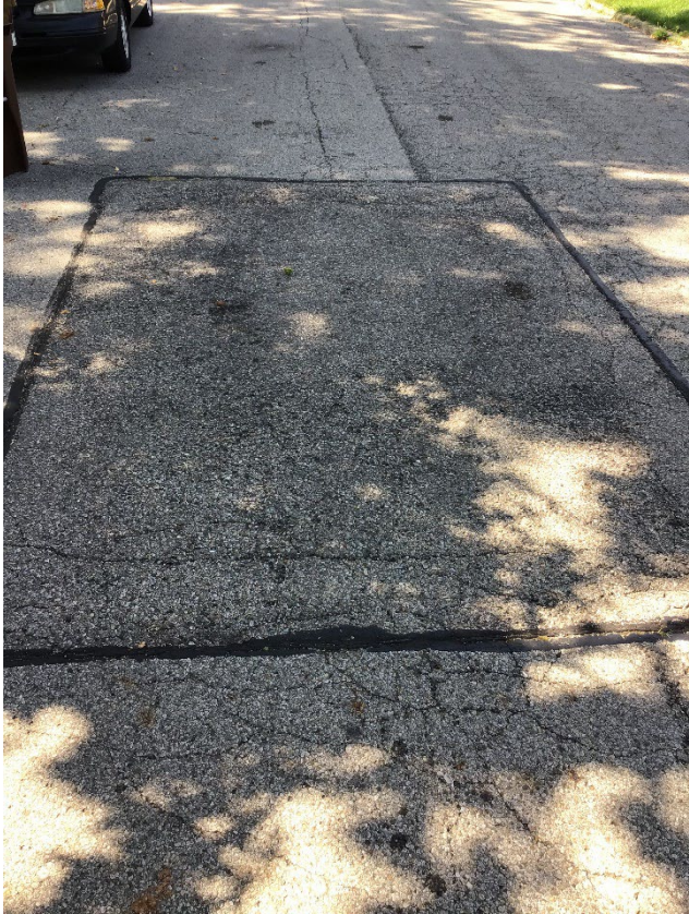
Rio Ln patch, facing west
