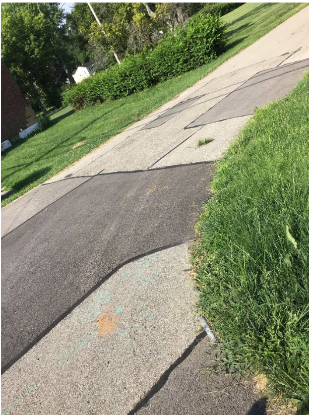
Imperial Ave patches, facing west
