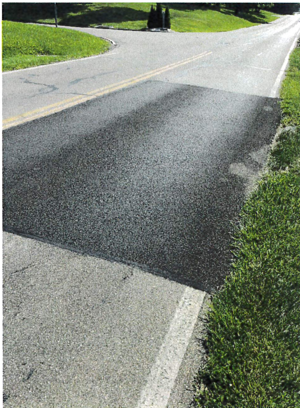
Rahn Road patch, facing east
