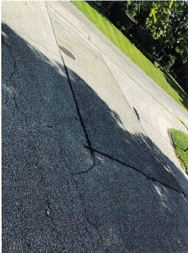
Silbury Lane patch, facing north
