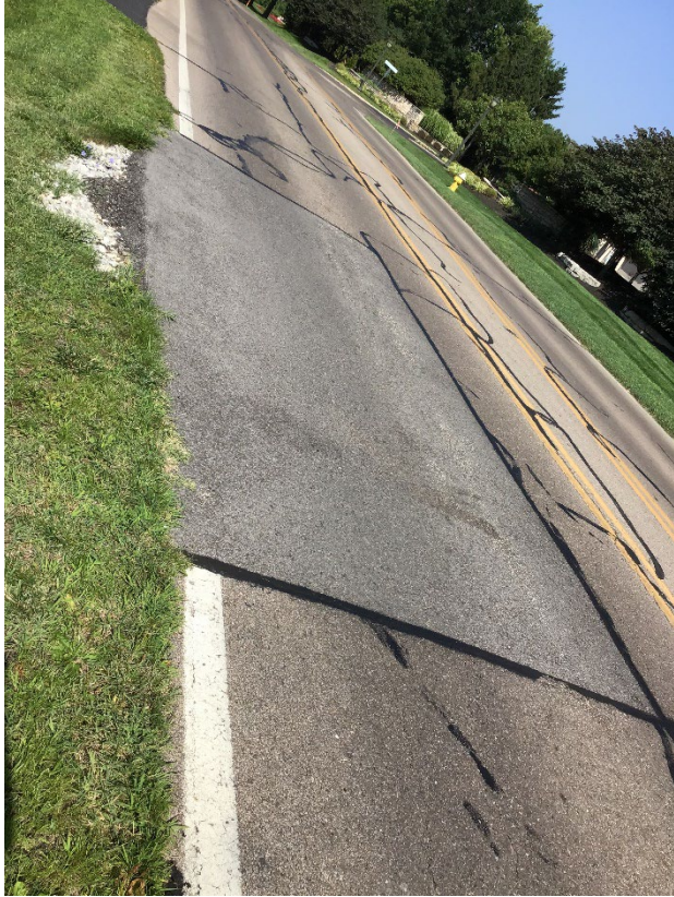
Rahn Road patch, facing east
