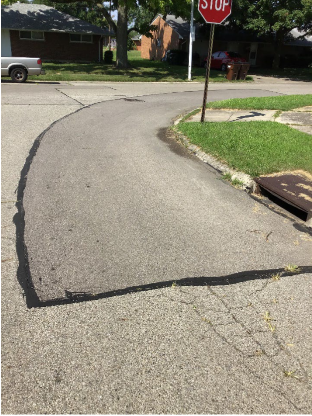
Chee Ct patch, facing southwest
