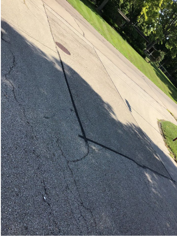
Silbury Lane patch, facing north
