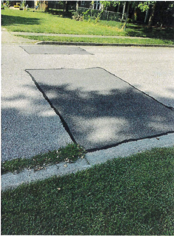
Eldorado Ave patches, facing west
