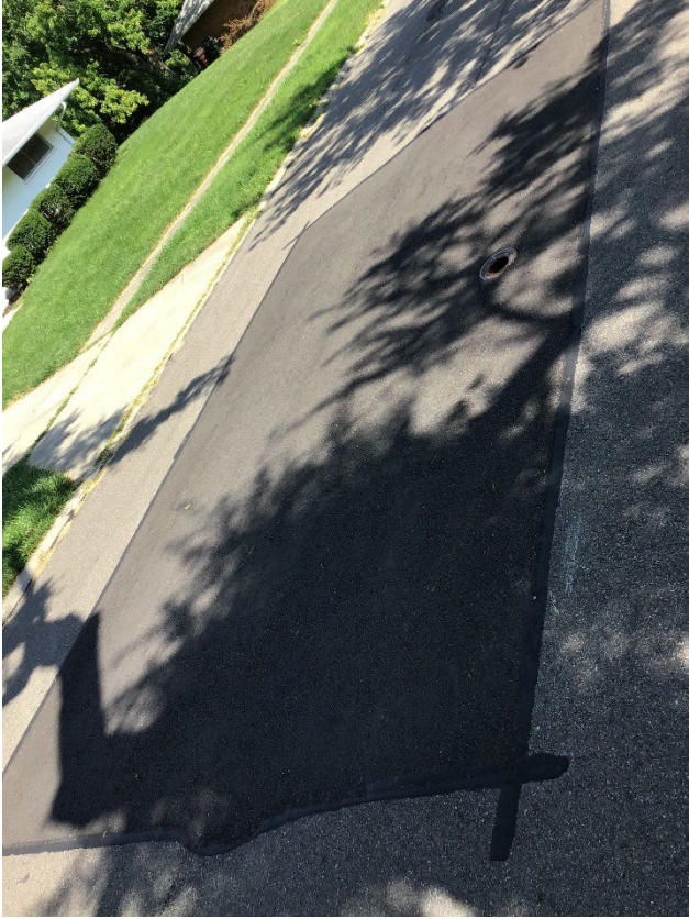
Sunray Rd patch, facing north
