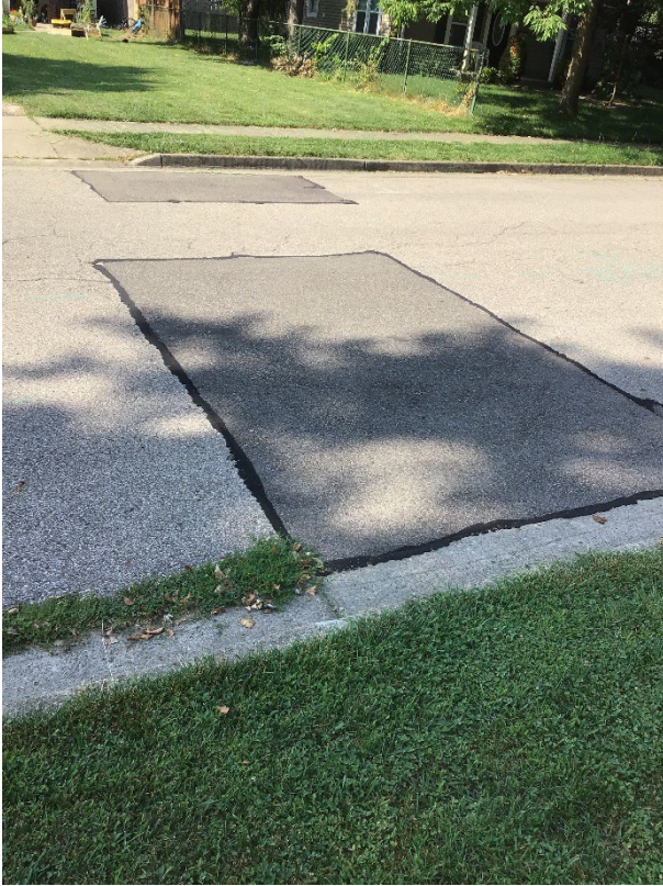
Eldorado Ave patches, facing west
