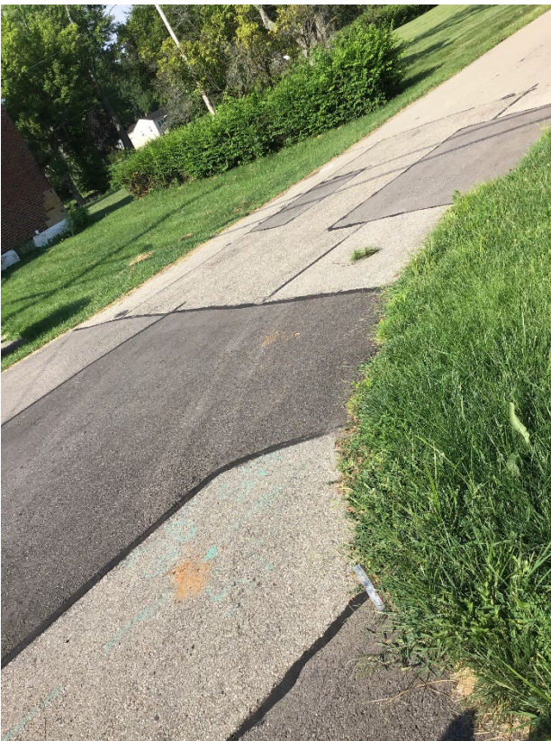
Imperial Ave patches, facing west
