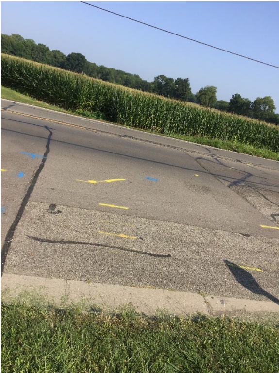
Brandt Pike patches, all facing northeast
