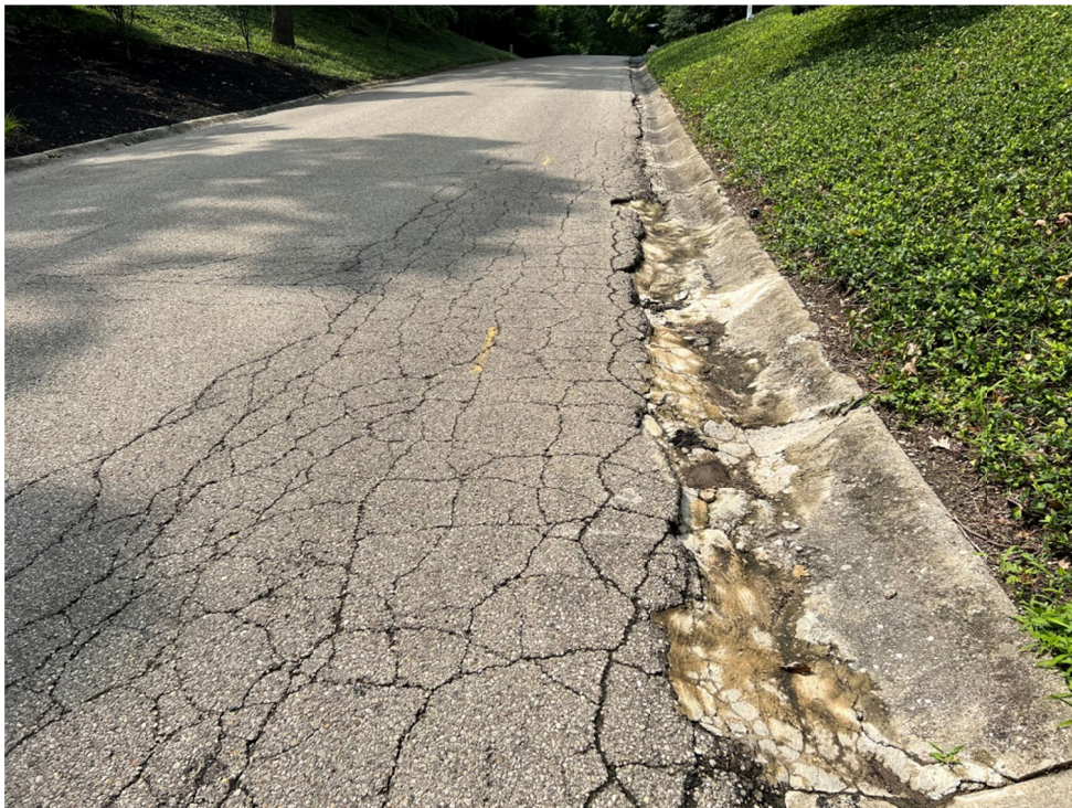
Southern Boulevard, facing south. Cracking asphalt pavement exacerbated by deteriorated curb.
