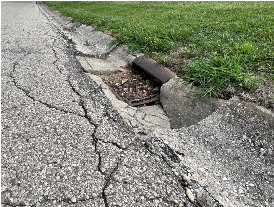
Southern Boulevard, facing north. Cracking asphalt pavement exacerbated by failed catch basin.
