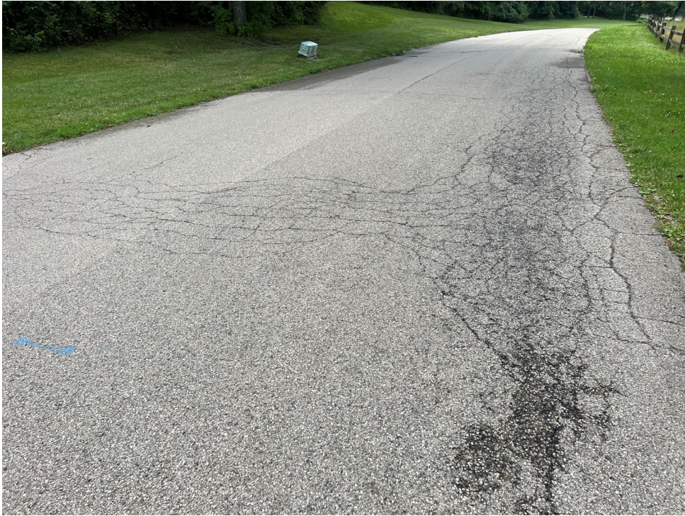
Southern Boulevard, facing south. Deteriorating asphalt pavement surface. Remaining curb mostly overgrown with vegetation.
