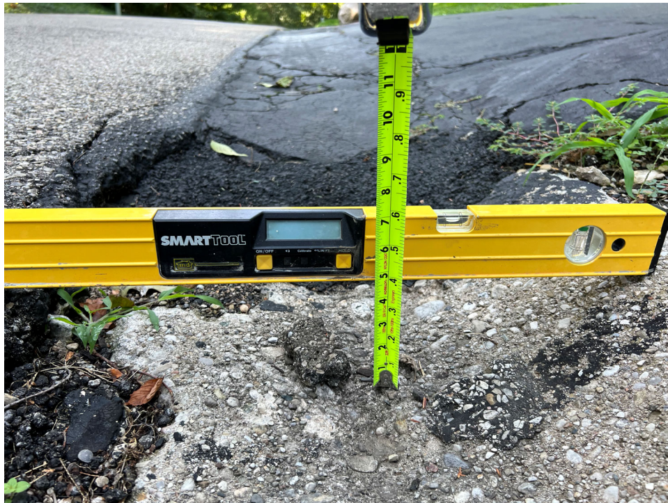
Southern Boulevard, facing south. Curb gutter more than 4 inches low (half inch typical).
