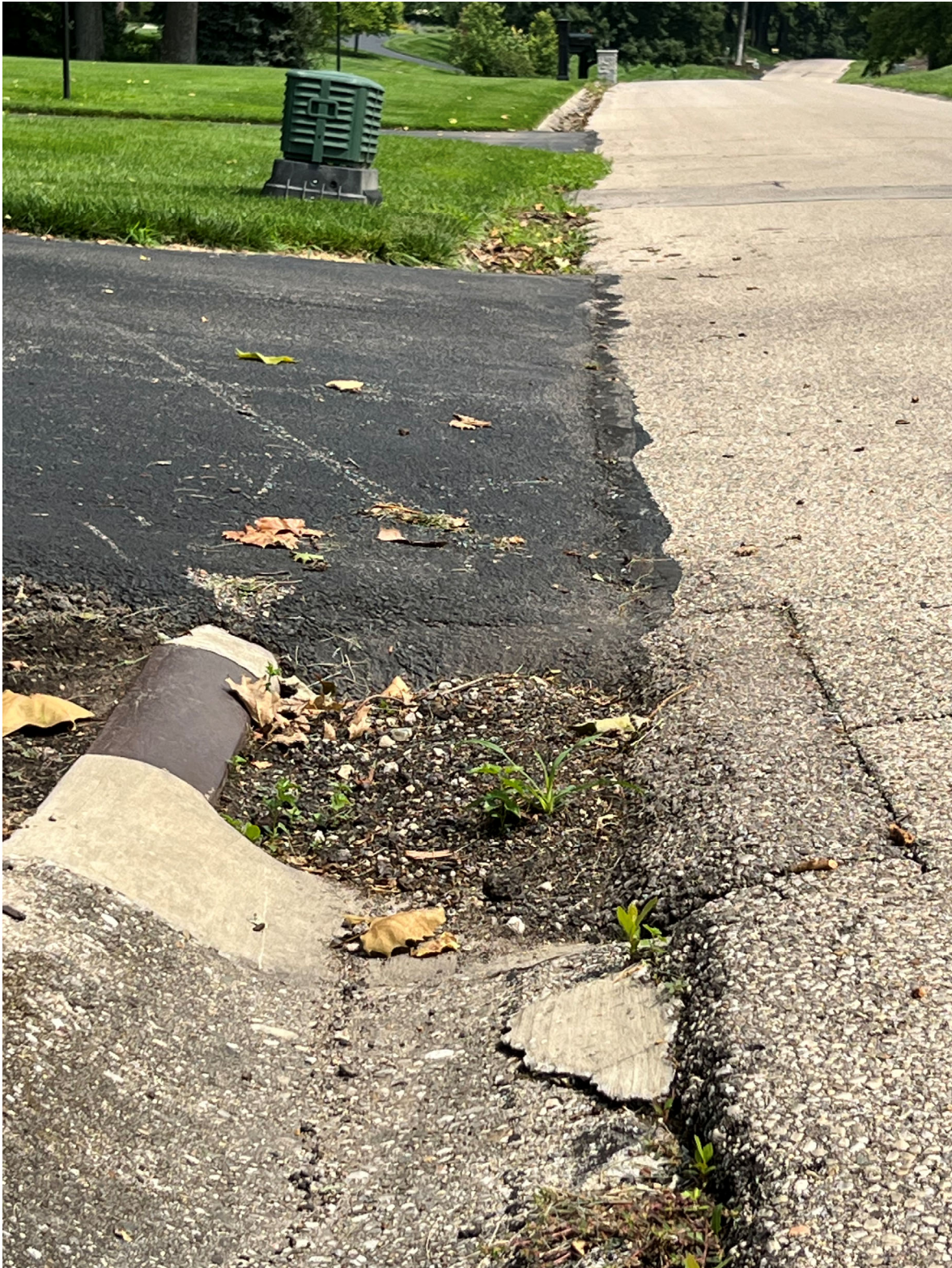
Southern Boulevard, facing north. Asphalt edge unsupported and falling towards catch basin and gutter. Gutter filled with asphalt at driveway and grass beyond that.
