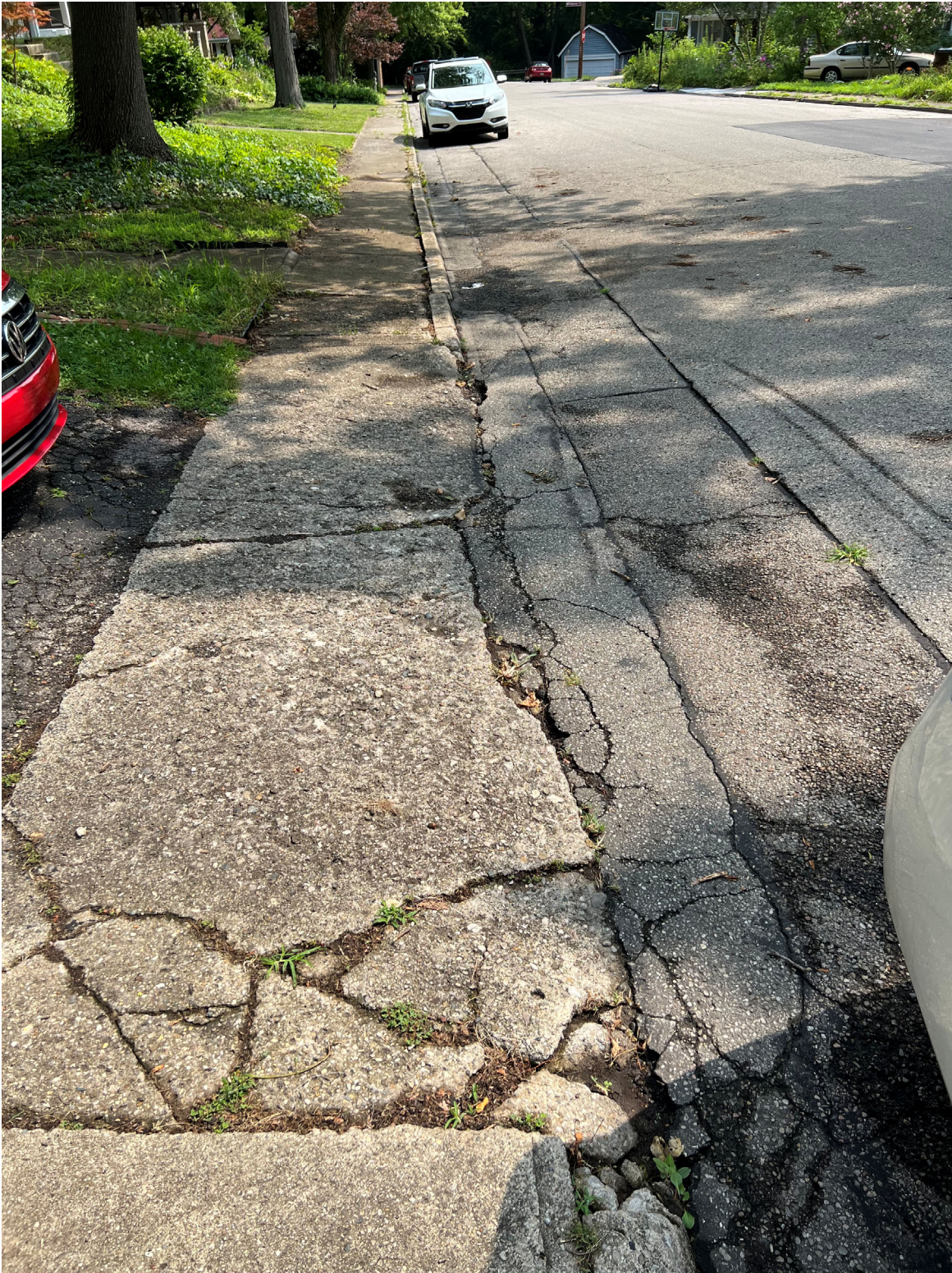
Southern Boulevard, facing north. Asphalt patching and cracking. Gutter paved over with asphalt in past to cover gutter and provide additional pavement thickness. Deteriorated drive approach, sidewalk and curb.
