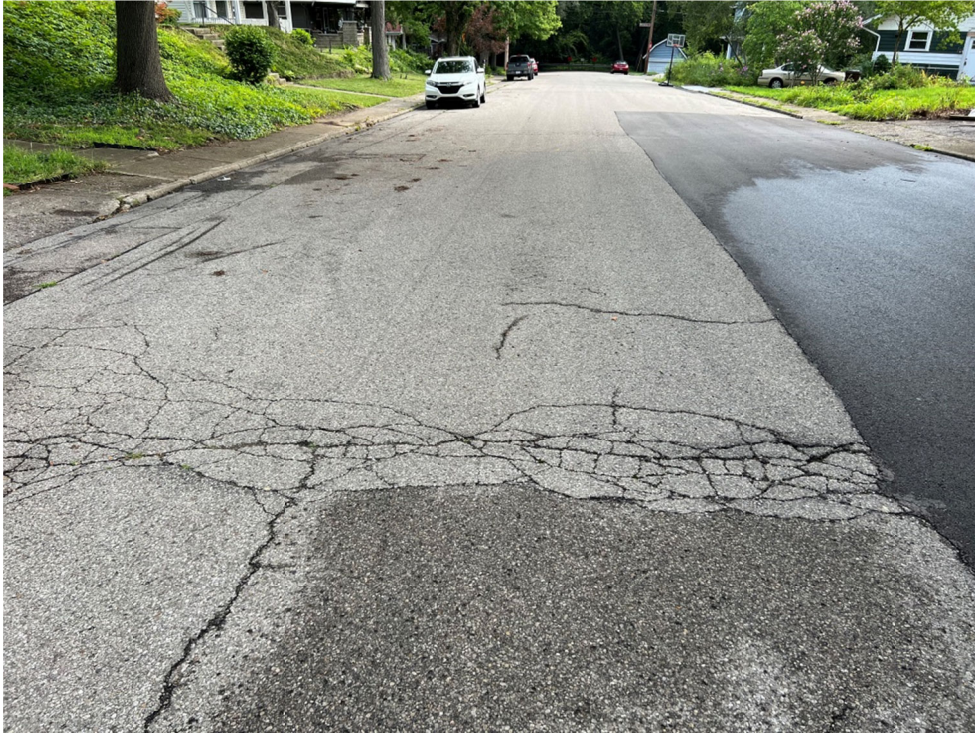
Heritage Point Drive, facing north. Deteriorating asphalt pavement surface – worst was already patched. Street is overly wide for traffic. Cross-slope out of spec for sidewalks at the back of curb – mostly due to tree roots.
