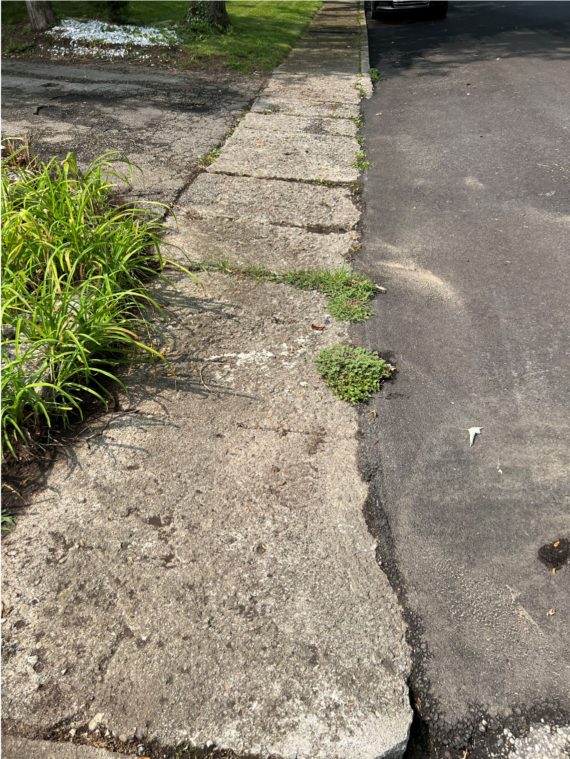
Southern Boulevard, facing south. Asphalt patching. Deteriorated drive approach, sidewalk and curb.
