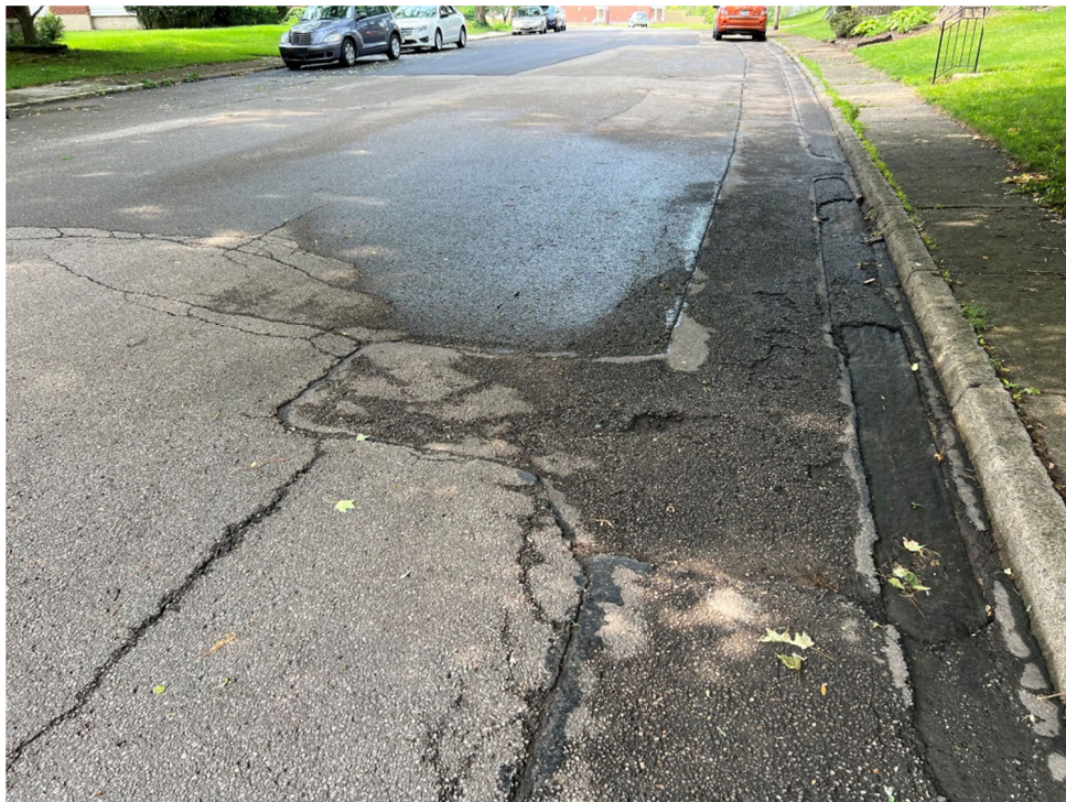
Heritage Point Drive, facing south. Cracking and missing asphalt pavement exacerbated by deteriorating gutter.
