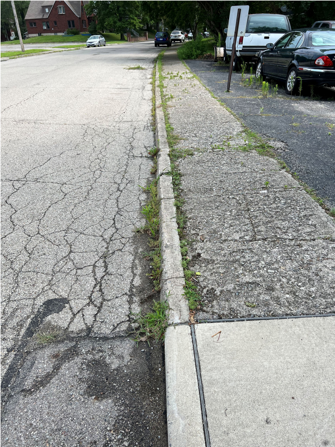
Southern Boulevard, facing north. Significant cracking of asphalt. Deteriorating curb and sidewalk.
