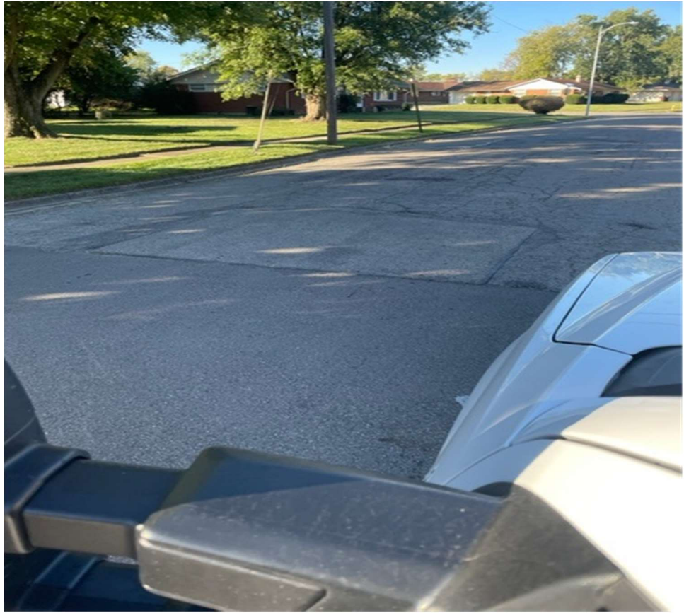
717-720 MacMillan Drive (2 Water Main Breaks)
