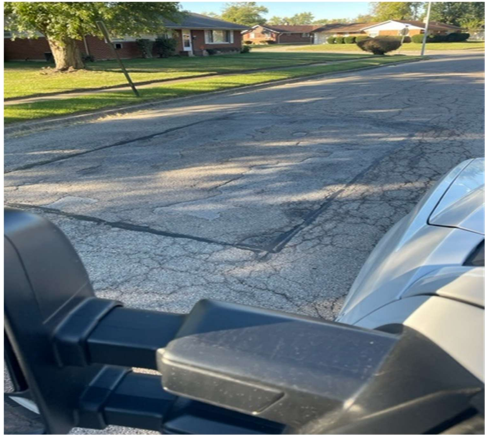
701 MacMillan Drive (1 Water Main Break)
