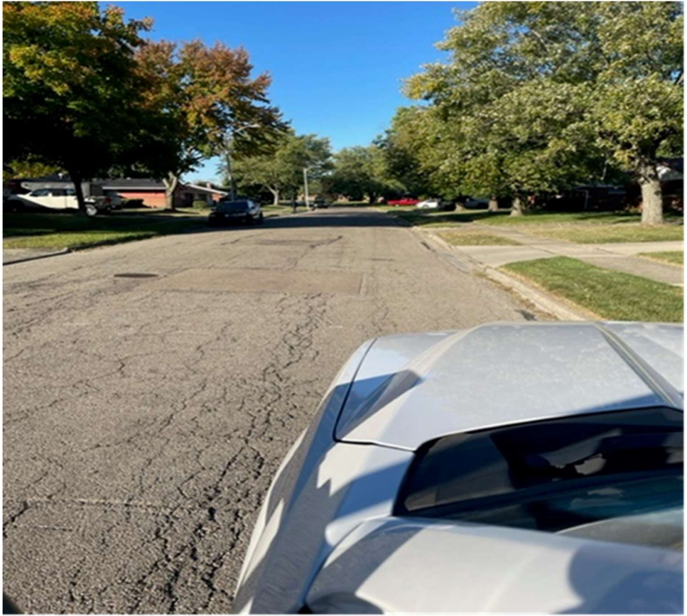
800 MacMillan Drive (1 Water Main Break)
