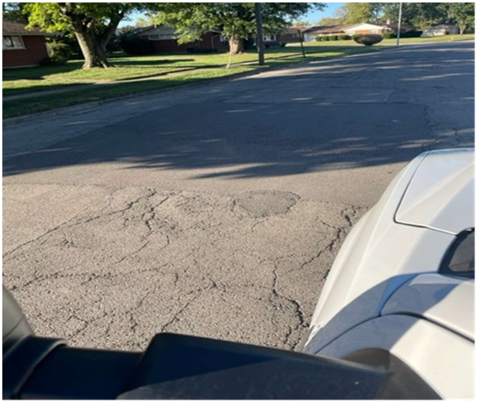
712 MacMillan Drive (3 Water Main Break)
