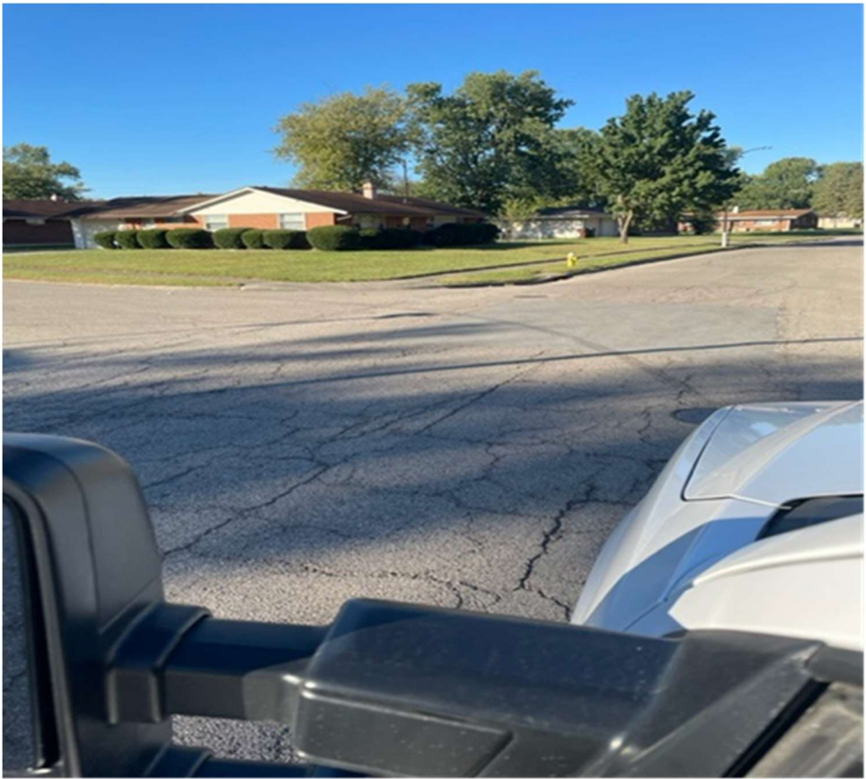
627 MacMillan Drive (1 Water Main Break)
