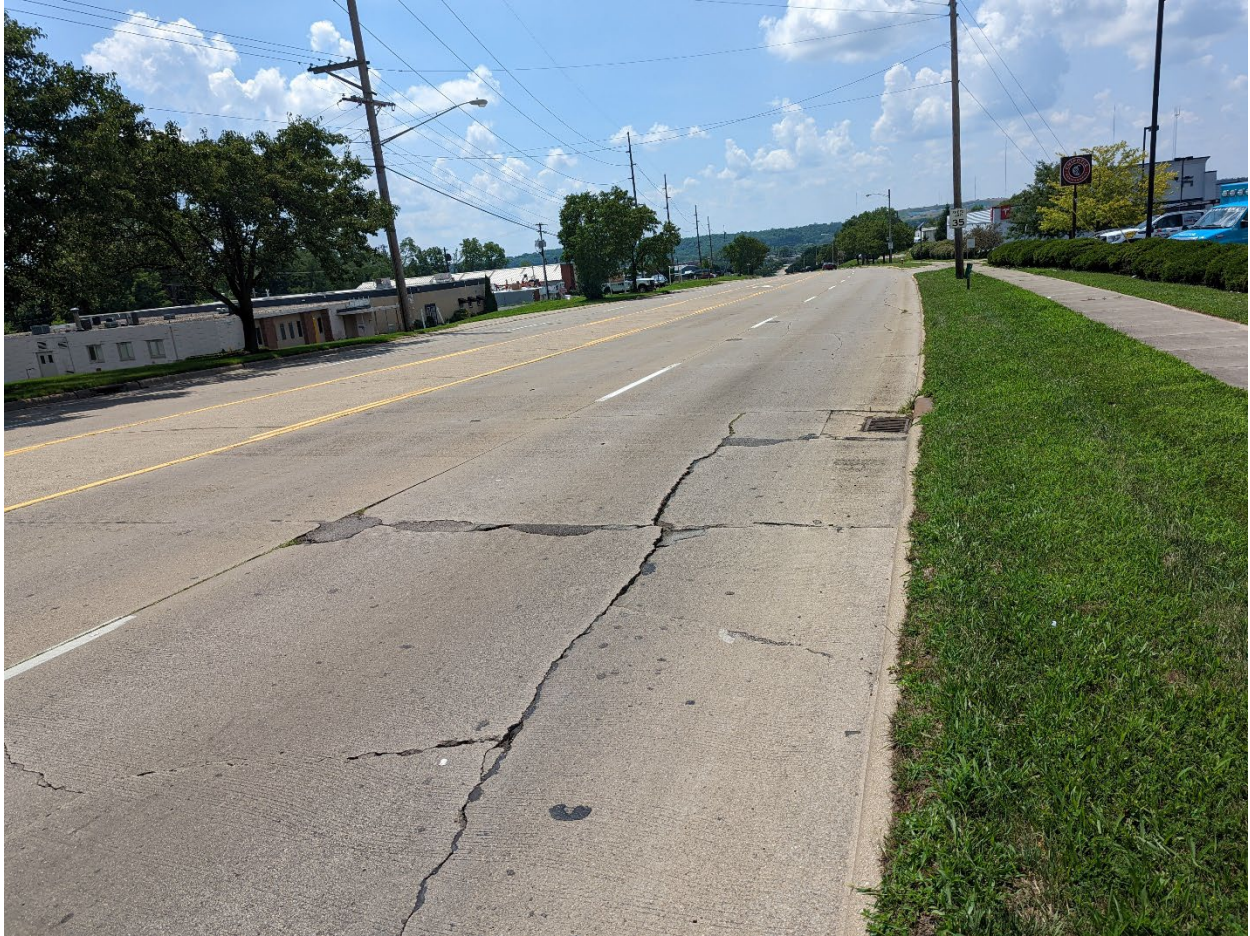
Figure 1: Deteriorated and Patched Pavement
