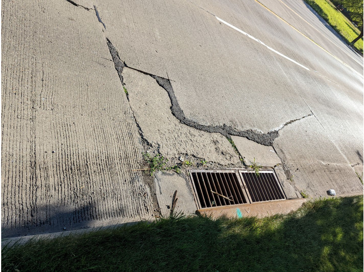
Figure 4: Cracking and Patched Pavement
