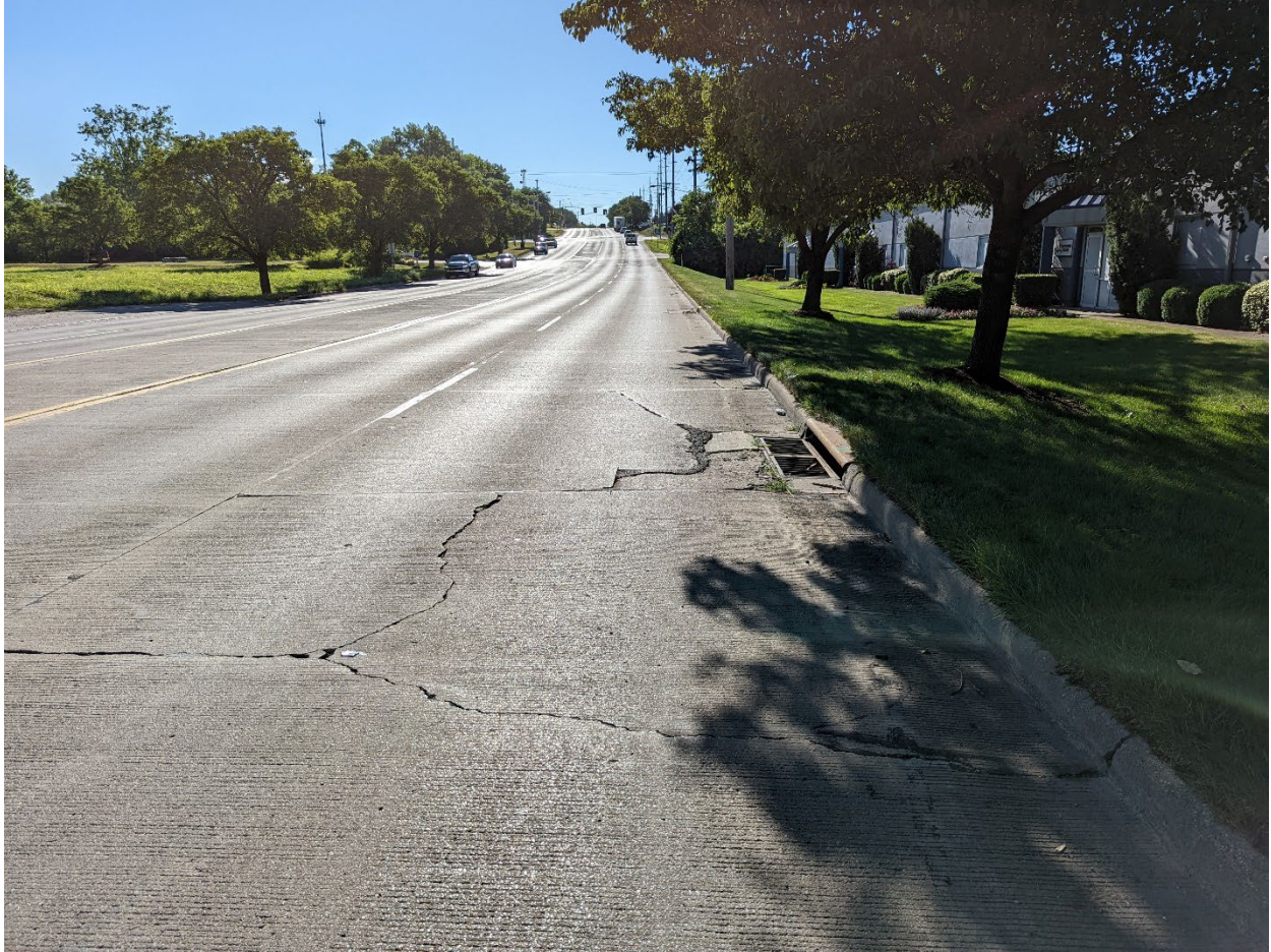
Figure 5: Longitudinal and Transverse Cracking
