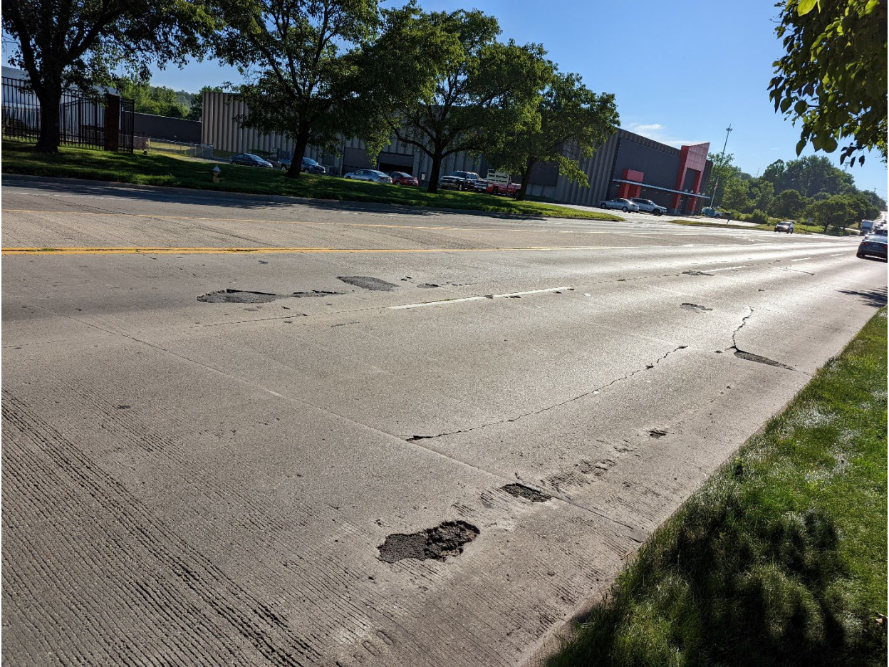
Figure 6: Longitudinal Cracking and Pot Holes
