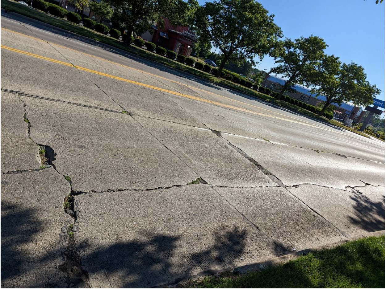
Figure 2: Severe Cracking, Potholes
