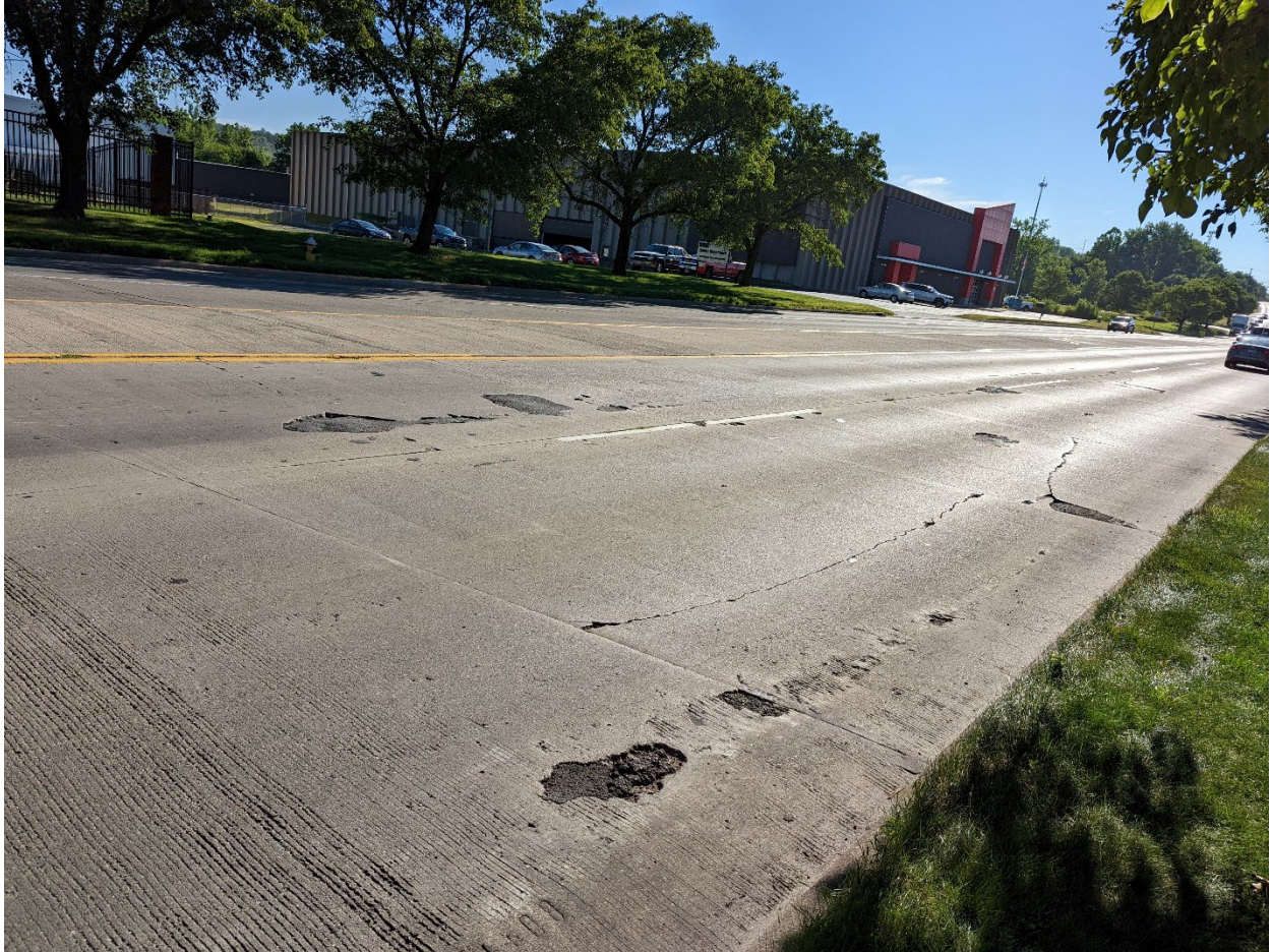
Figure 6: Longitudinal Cracking and Pot Holes
