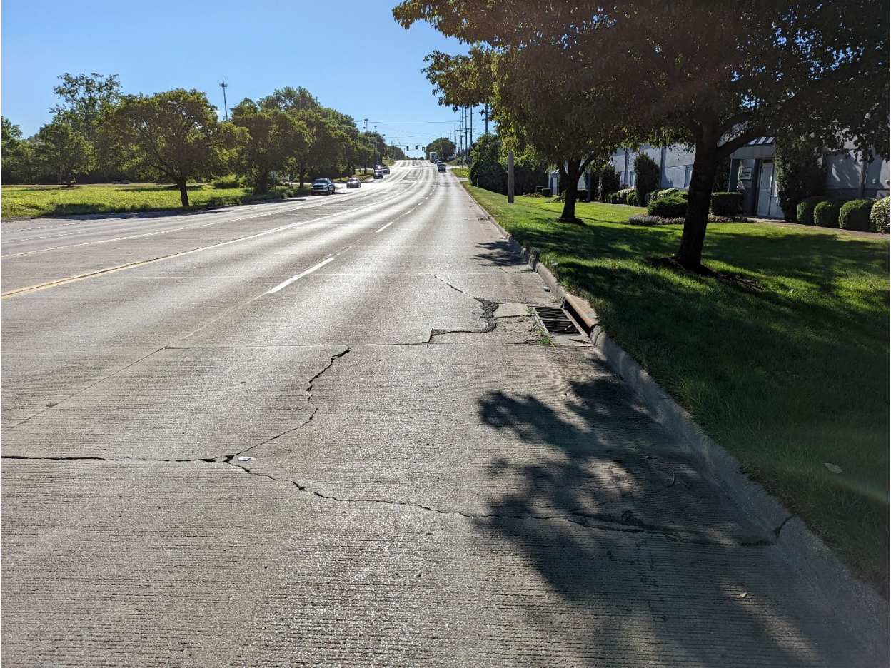
Figure 5: Longitudinal and Transverse Cracking
