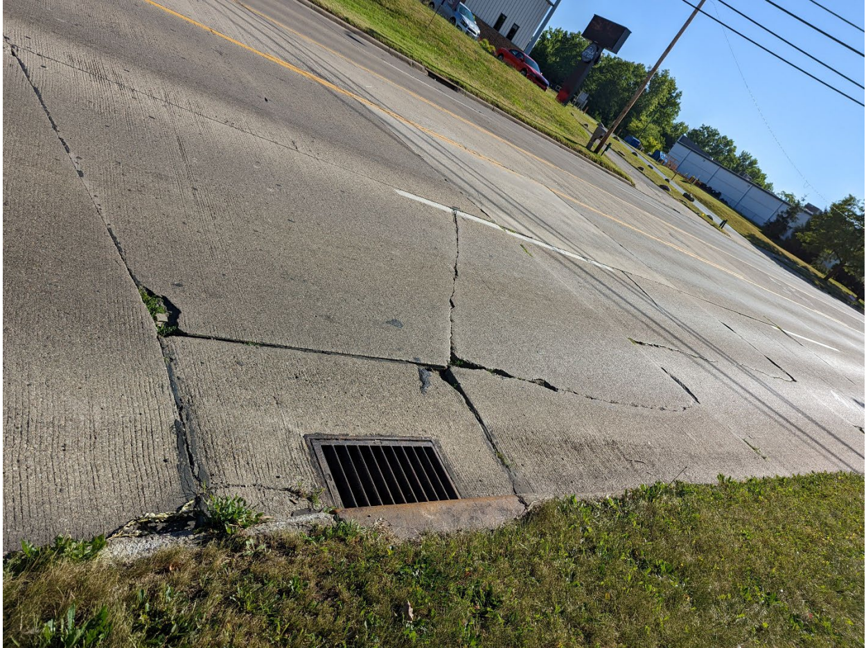
Figure 3: Longitudinal and Transverse Cracking
