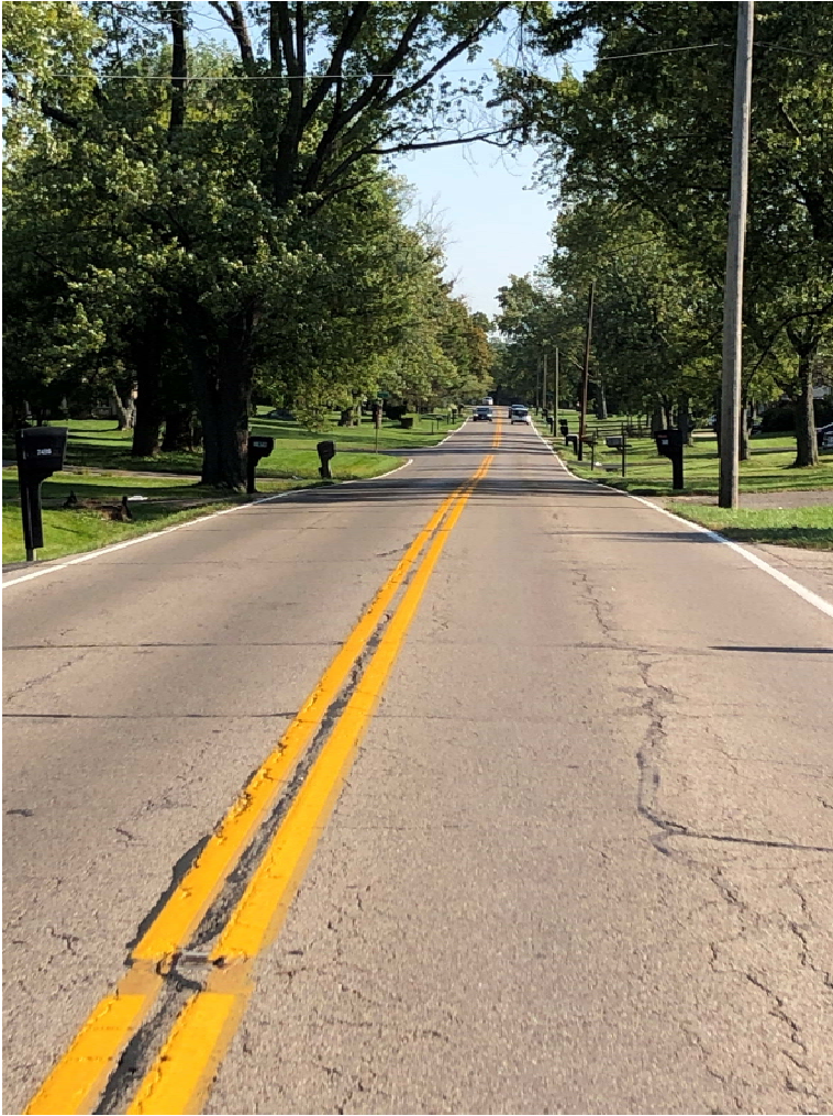
Looking north along Mad River Road Approximately 220 ft south of Bellsburg Dr.
