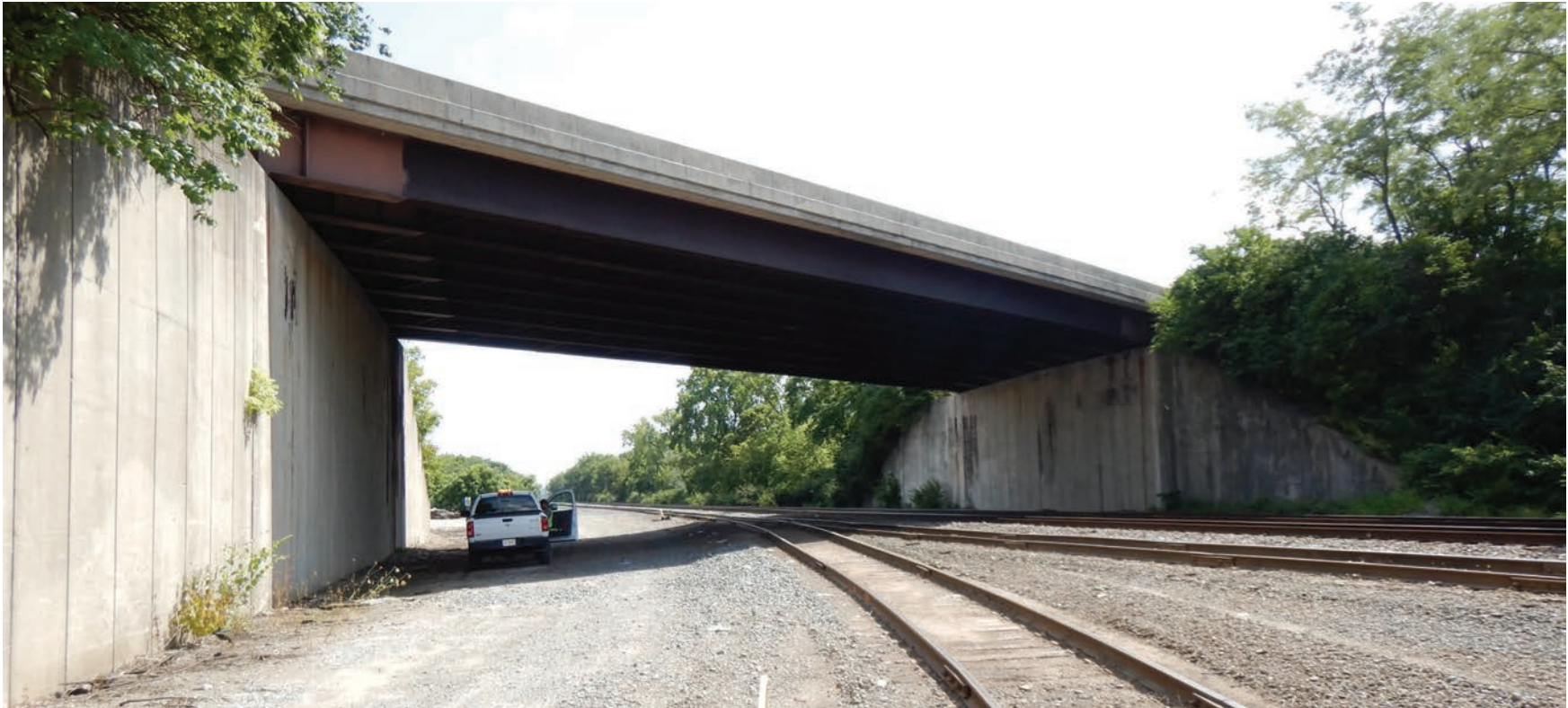
Profile View of the Wagner Ford Road Bridge over the CSX Railroad as seen from the North Looking South
