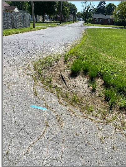
Alligator cracking and pothole on Comer Ct.
