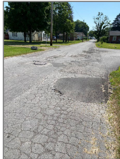
Alligator Cracking and potholes on Comer Ct.
