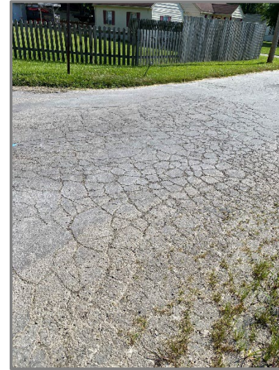
Alligator Cracking on Comer Ct.
