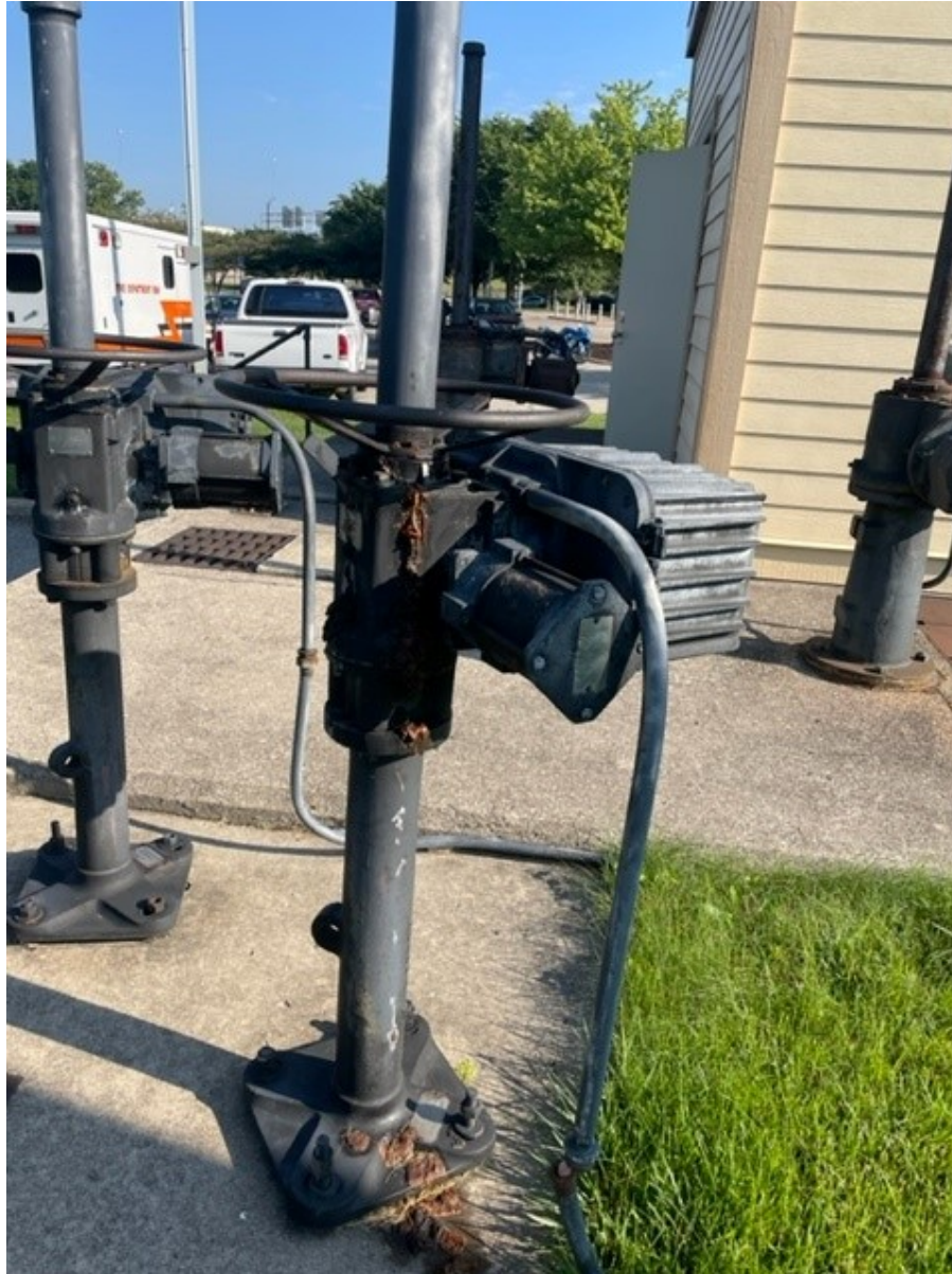
Figure 3 - Three (3) of the existing actuators
