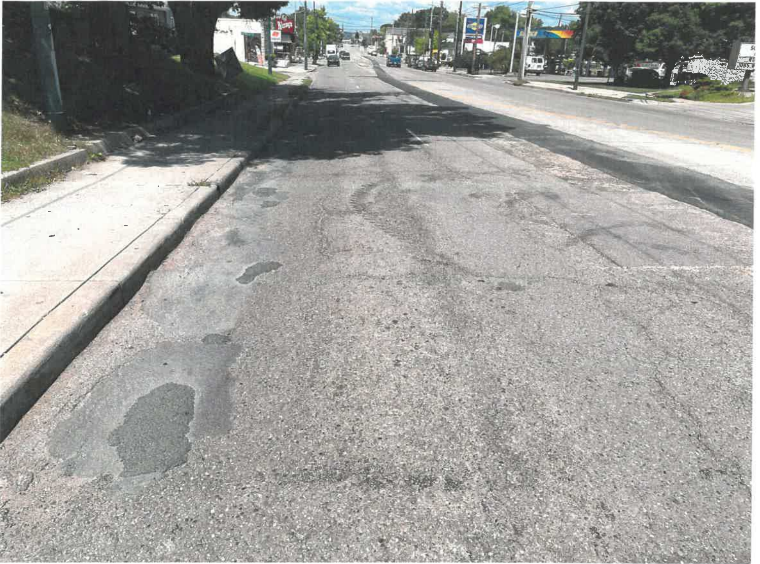
Cracking with patches on Wayne Avenue
