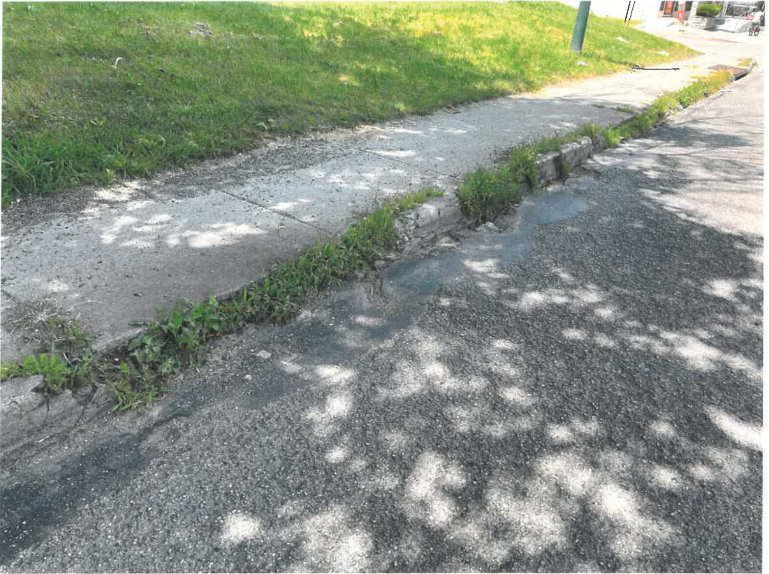
Cracked and broken curb on Wayne Avenue
