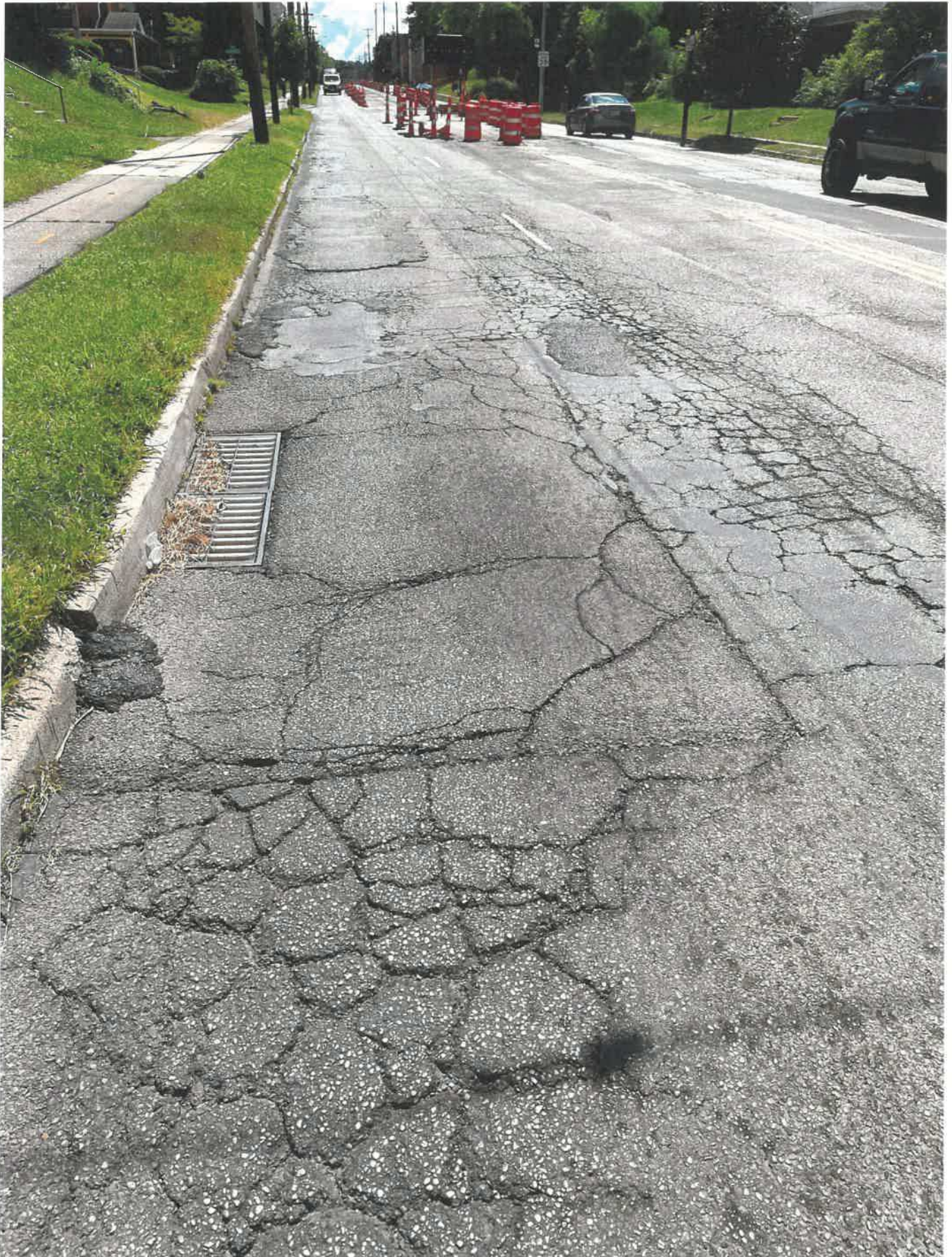
Cracked, broken, and patched pavement on Wayne Avenue
