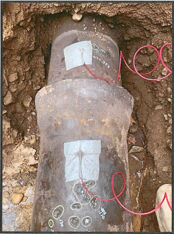
Dig 3 Pipe Test Leads
