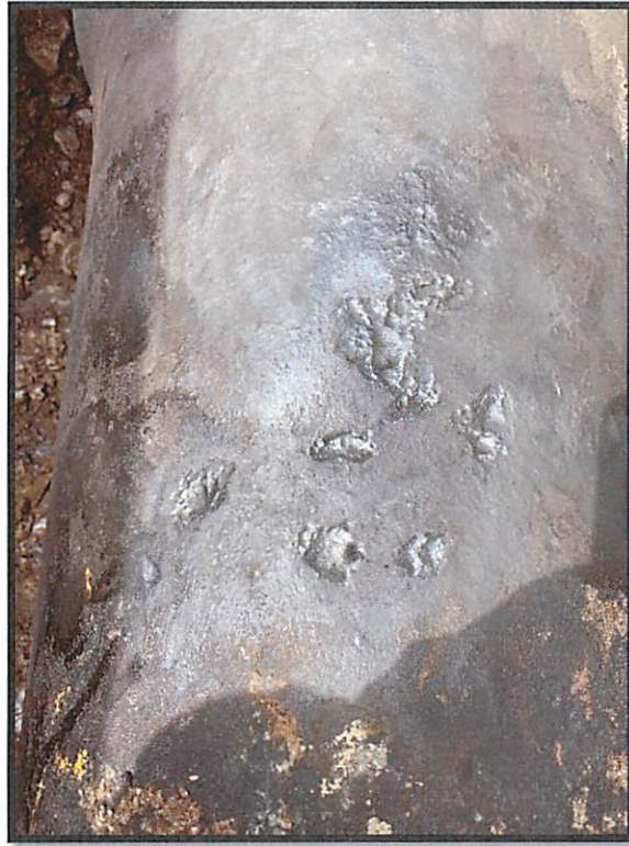
Pitting revealed after cleaning
