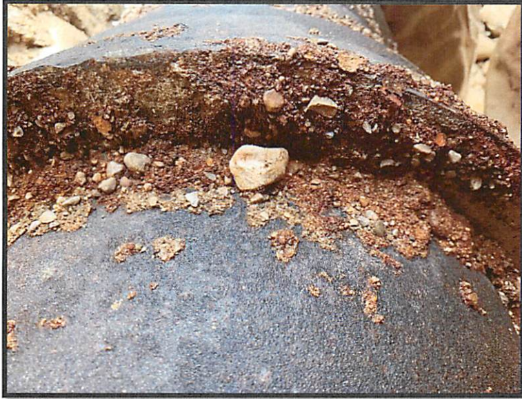
Magnetite at Dig 3 joint
