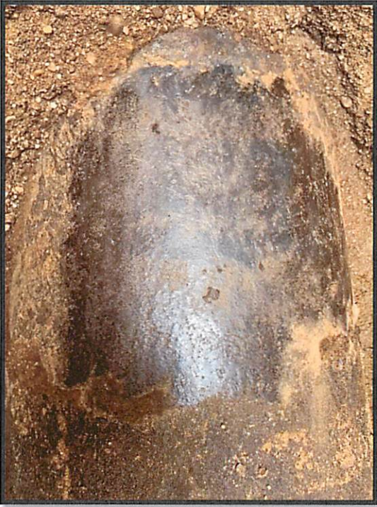
Dig Site 2 negligible uniform pitting
