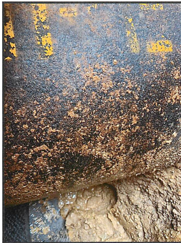
Dig Site #1 Visible paint from manufacturer
