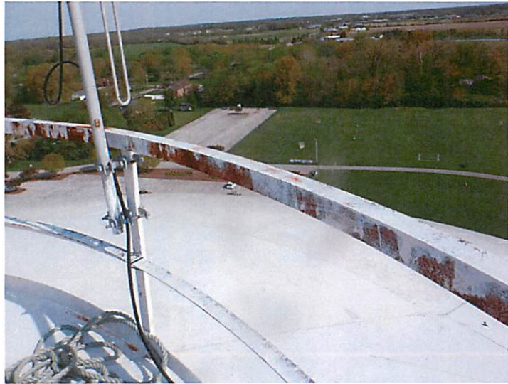
26) The roof handrail is in good condition. There are coating failures on the railing.
