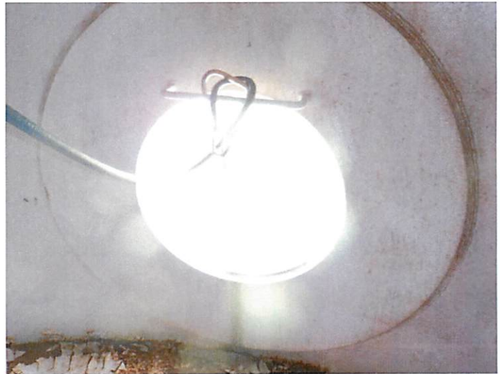
50) The painter's hatch at the top of the riser is in good condition. There is a handhold over the opening.
