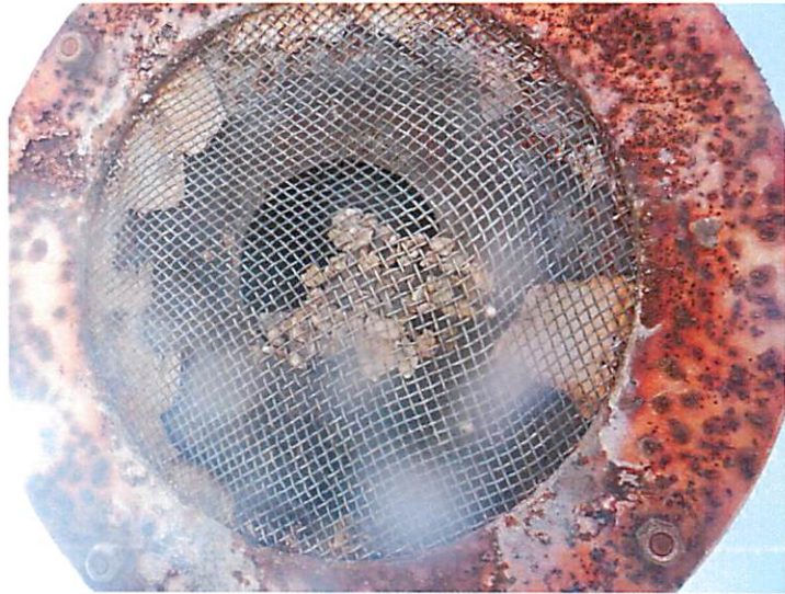
8) The overflow screen is in good condition. There are coating failures on the flange.
