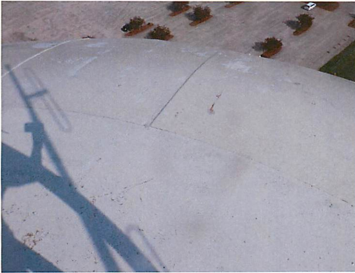
16) The coating on the roof is in fair condition with moderate failures.
