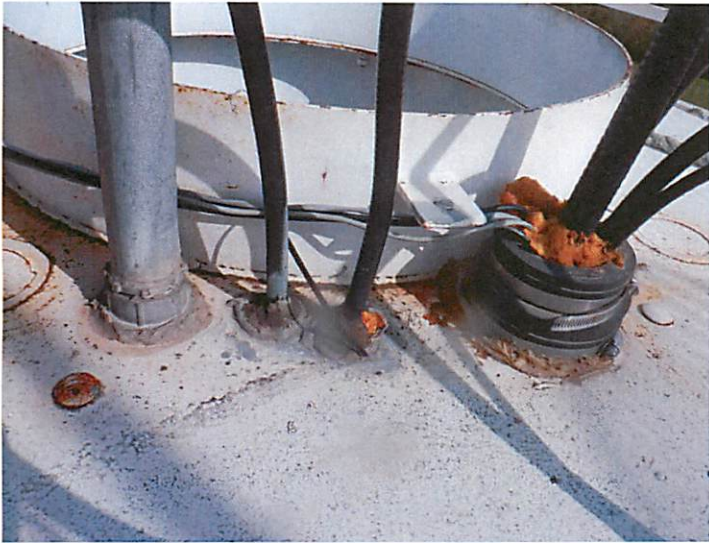
28) The roof cable penetrations are sealed with caulk and spray foam.
