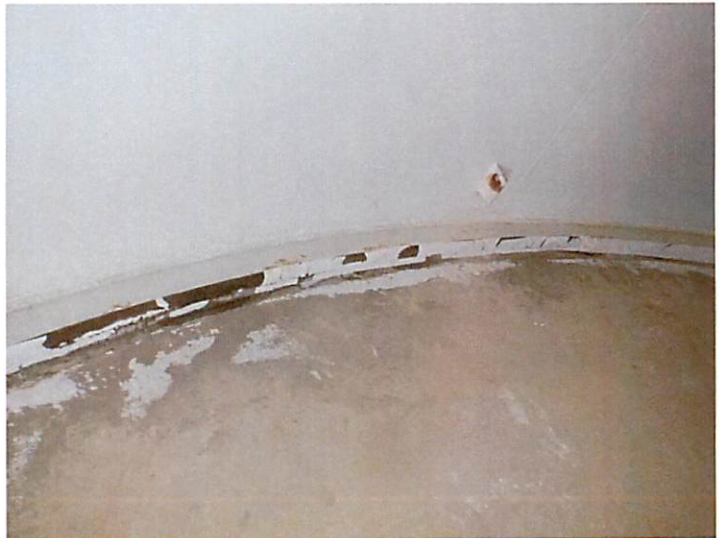
35) The basebell coating is in good condition with delamination on the baseplate.
