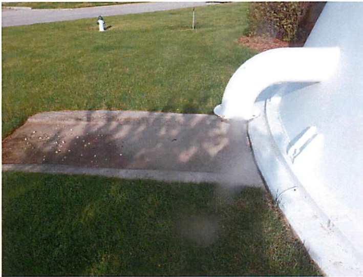
7) The overflow pipe discharges to concrete splash pad.
