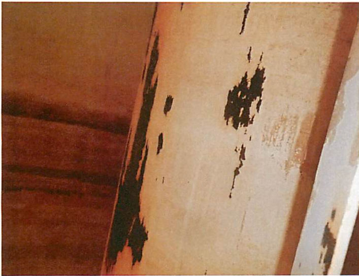
67) There is coating damage on the access tube likely from ice movement.
