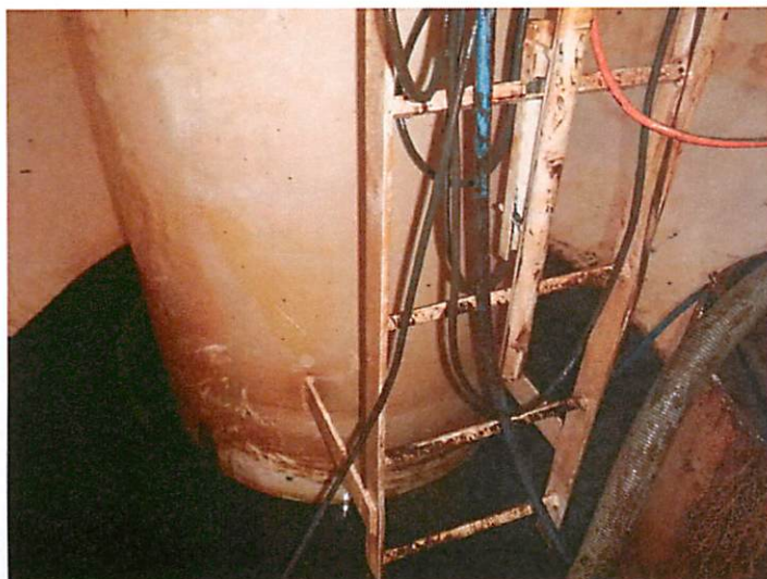
63) The wet interior ladder is in good condition. The ladder is equipped with a fall prevention device.
