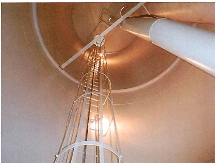
45) The riser ladder is in good condition. The ladder is equipped with a fall prevention device and is caged.
