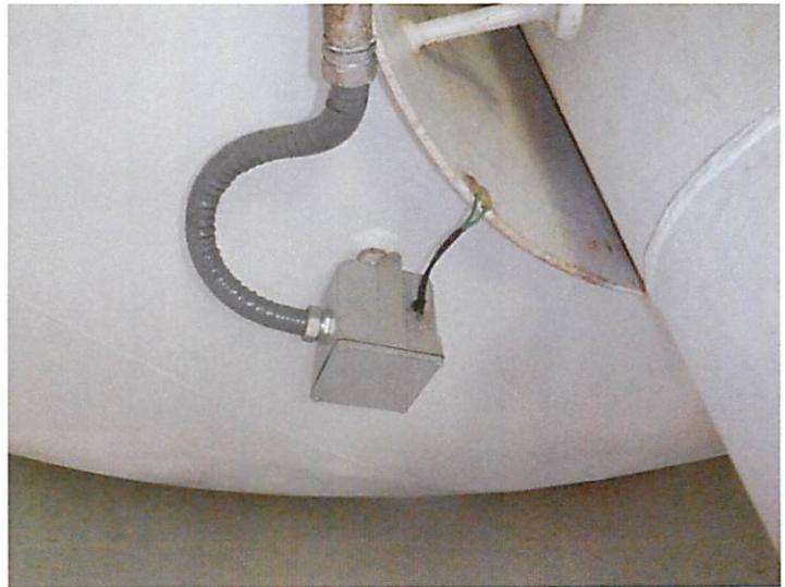
53) The pressure fitting for cathodic protection appears to be in good condition.
