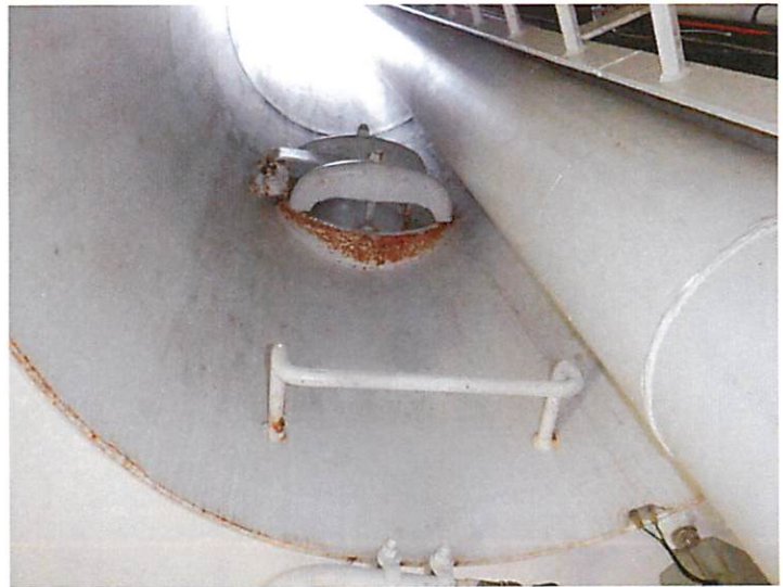
56) The wet interior manway located in the access tube is in good condition.
