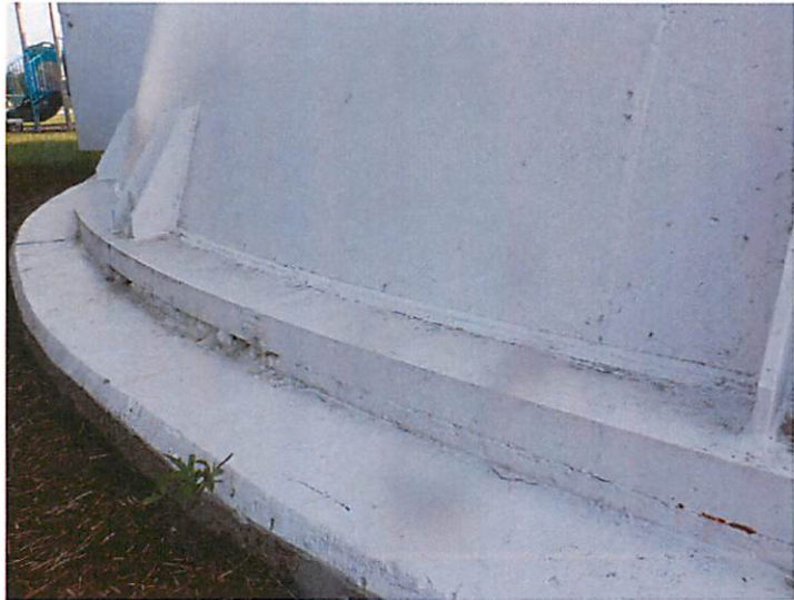
2) The grout between the steel foundation and the concrete baseplate is in good condition.
