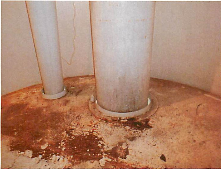
43) The condensate platform coating is in poor condition.
