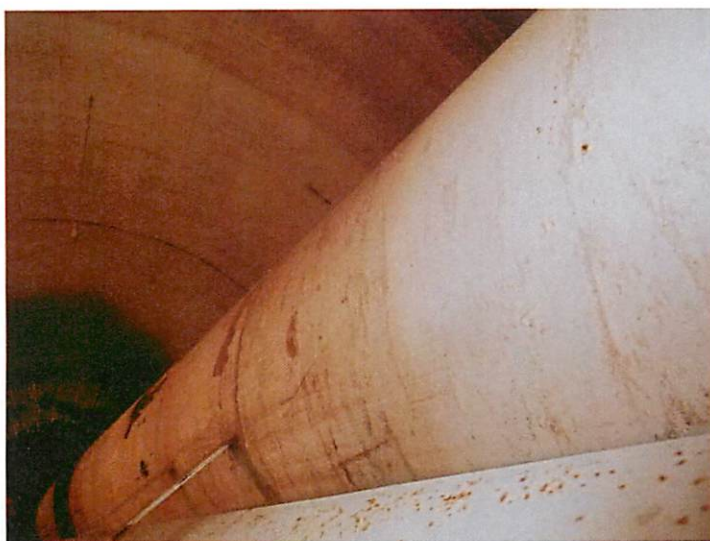
66) The coating on the access tube is in fair condition.
