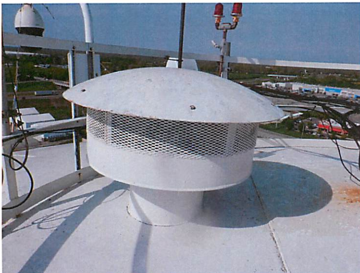
30) The roof vent is in good condition but there is no rain shield. The vertical expanded metal screen is in good condition.
