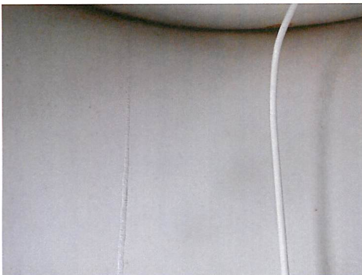
51) The coating on the riser above the top platform and the bowl is in good condition with minor failures.
