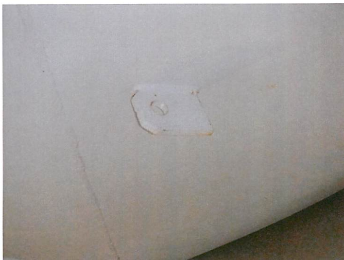
54) The rigging lug on the bowl above top platform hatch is in good condition.
