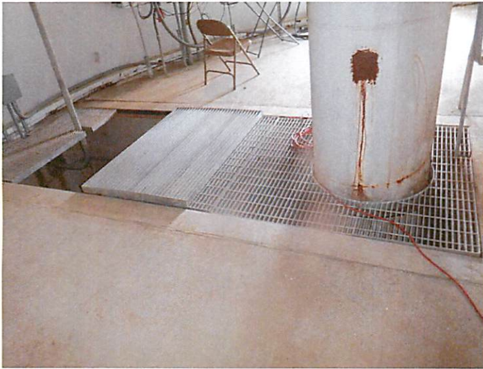
73) There is piping located in a pit in the basebell. The pit cover is in good condition.
