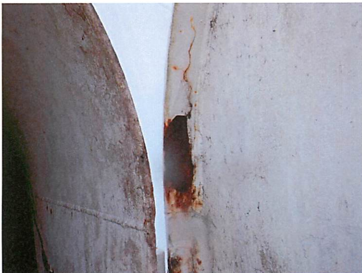
6) There are coating failures on the door.
