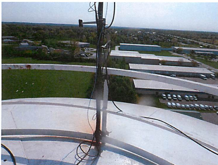
33) Antennas are mounted to the roof handrail.
