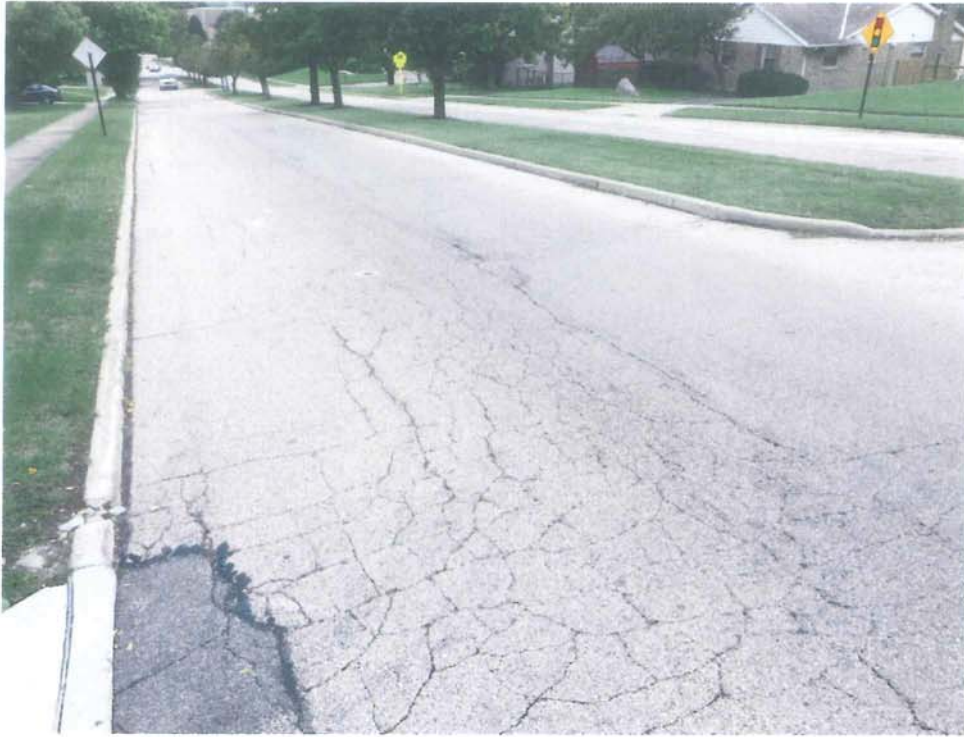
East David Road Looking Eastbound near Acreview Lane (deterioration of pavement and curb)
