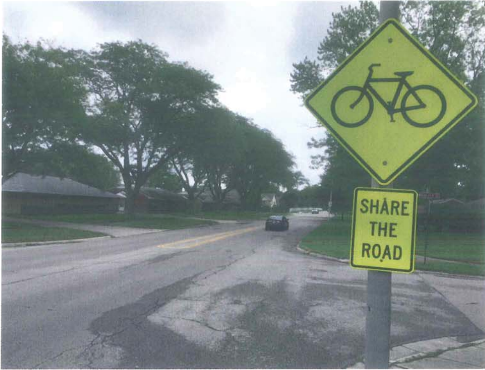
East David Road Looking Eastbound near Henrich Drive (deterioration of pavement, bike signage)
