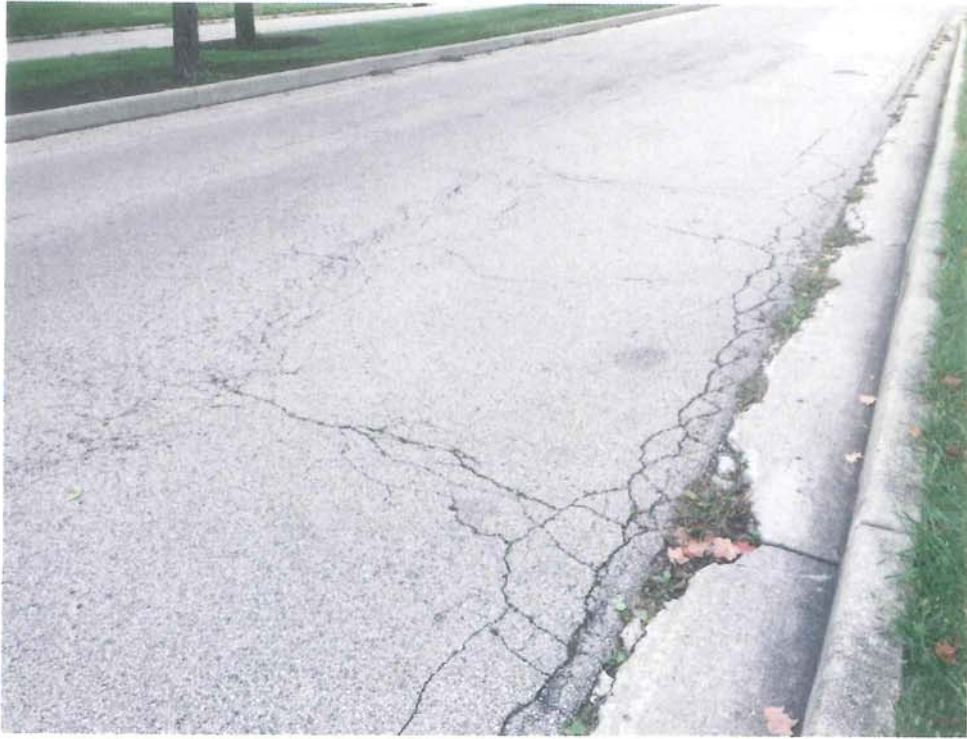
East David Road Looking Westbound near Wing View Lane (deterioration of pavement and curb)
