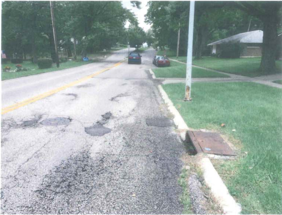
East David Road Looking Eastbound at Section of Proposed Improvement (narrowed lane to be widened for street bicyclists, deterioration of pavement and inlet)
