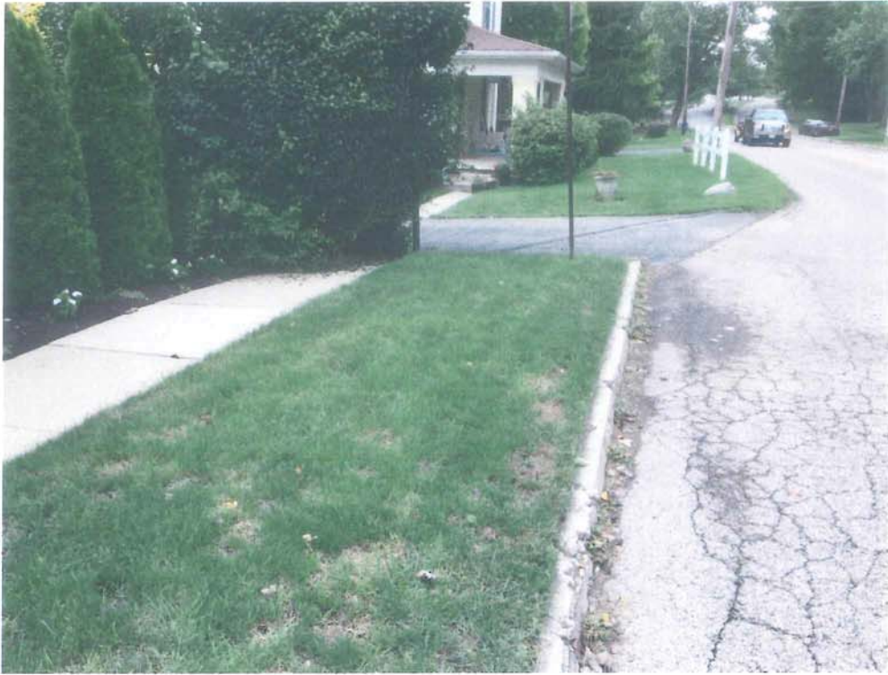
East David Road Looking Eastbound at Section of Proposed Improvement (termination of sidewalk and improved roadway, deterioration of pavement and curb)
