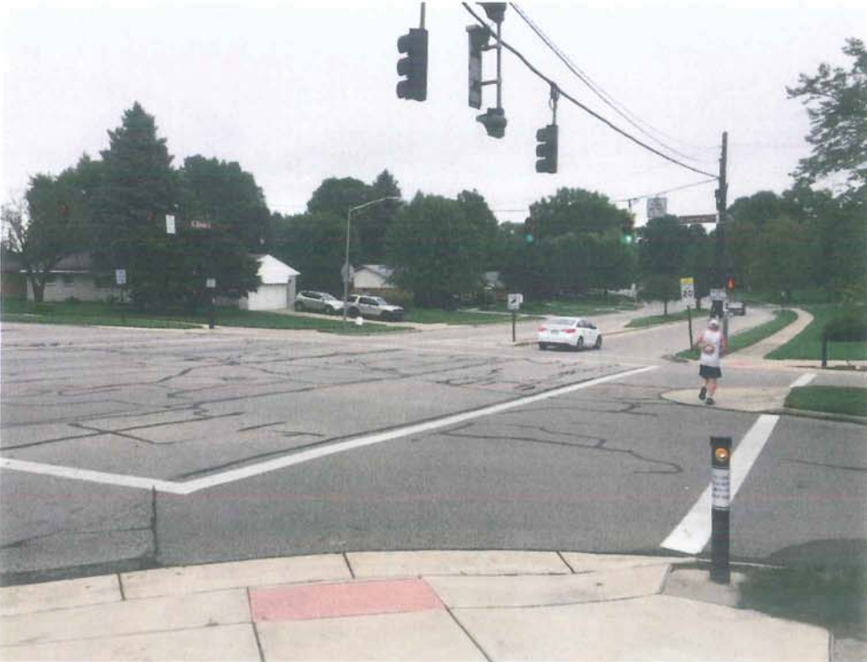
East David Road Looking Eastbound at Ackerman Boulevard (deterioration of pavement and curb, proposed traffic signal replacement)
