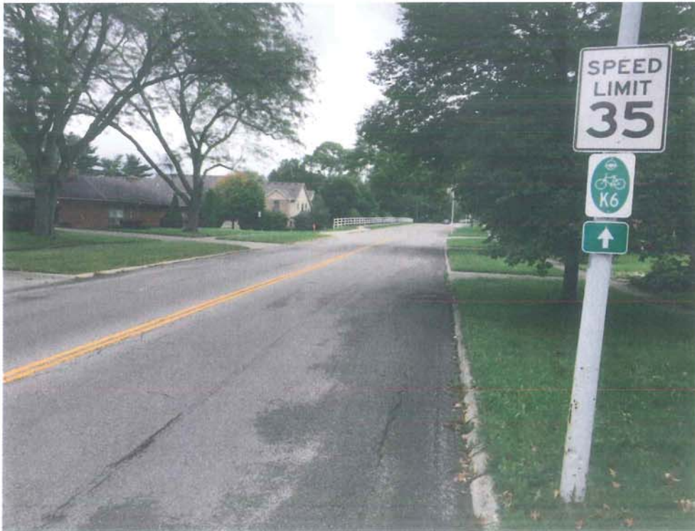
East David Road Looking Eastbound near Sunray Road (deterioration of pavement and curb, Kettering Bike Route K6)
