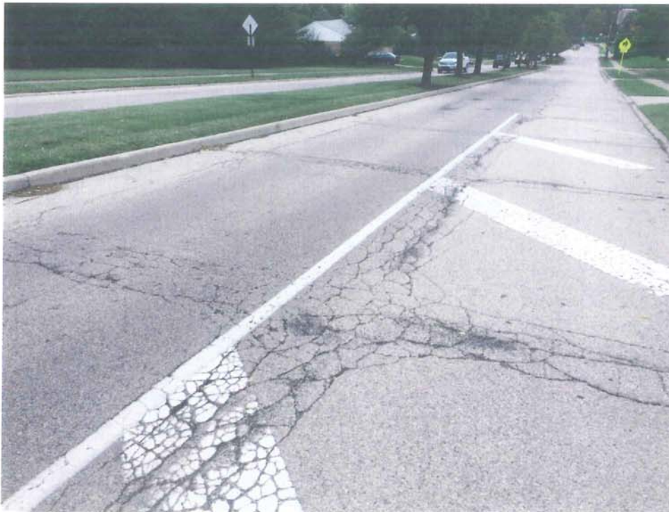
East David Road Looking Eastbound near Acreview Lane (deterioration of pavement and curb)
