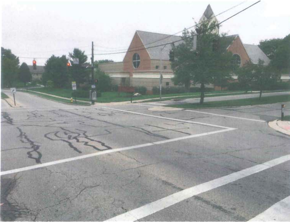
East David Road Looking Eastbound at Ackerman Boulevard (deterioration of pavement and curb, proposed traffic signal replacement)
