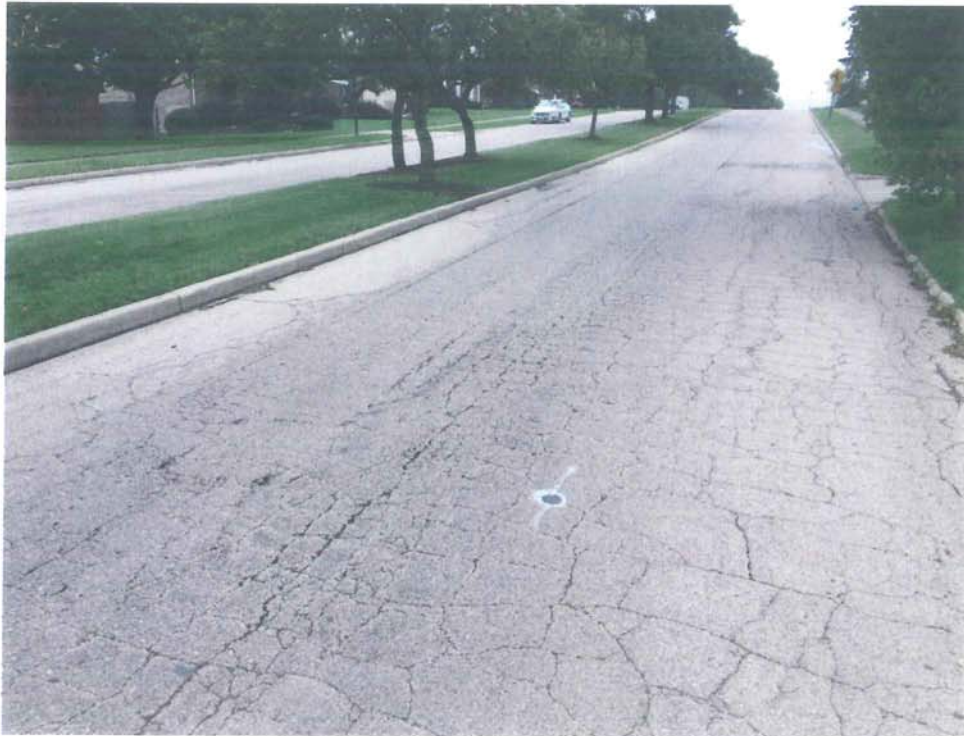
East David Road Looking Westbound near Wing View Lane (deterioration of pavement and curb)
