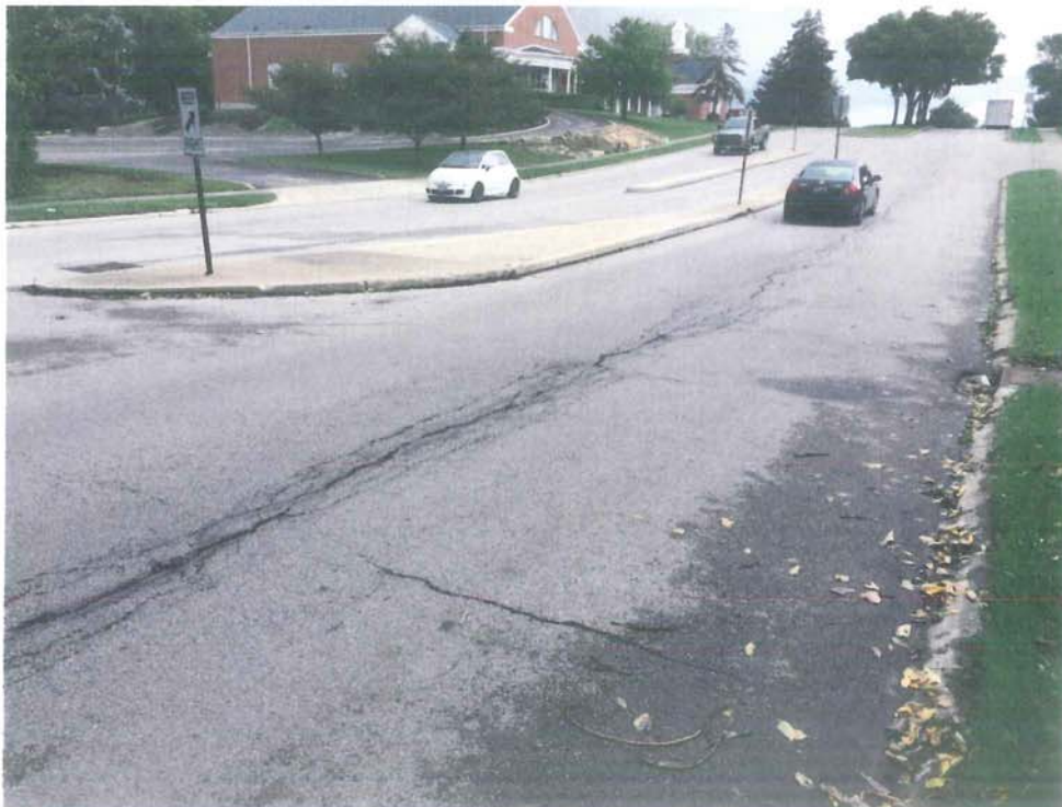
East David Road Looking Eastbound near Acreview Lane (deterioration of pavement, curb, and median)
