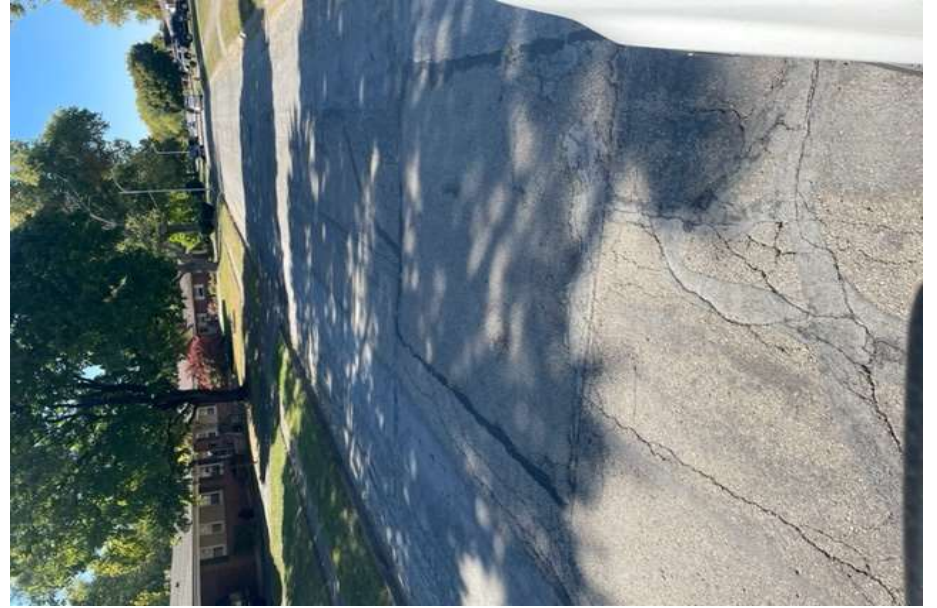
816 N. Eppington Drive (1 Water Main Break)
