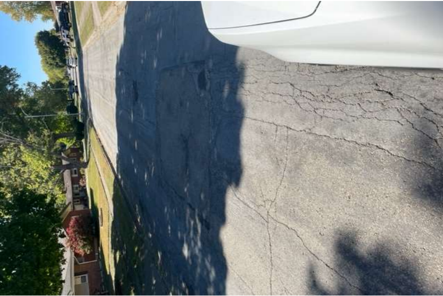
812 N. Eppington Drive (1 Water Main Break)
