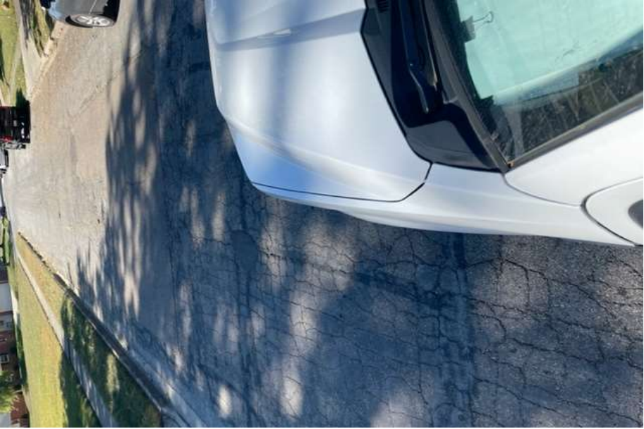
501 N. Eppington Drive (1 Water Main Break 1)
