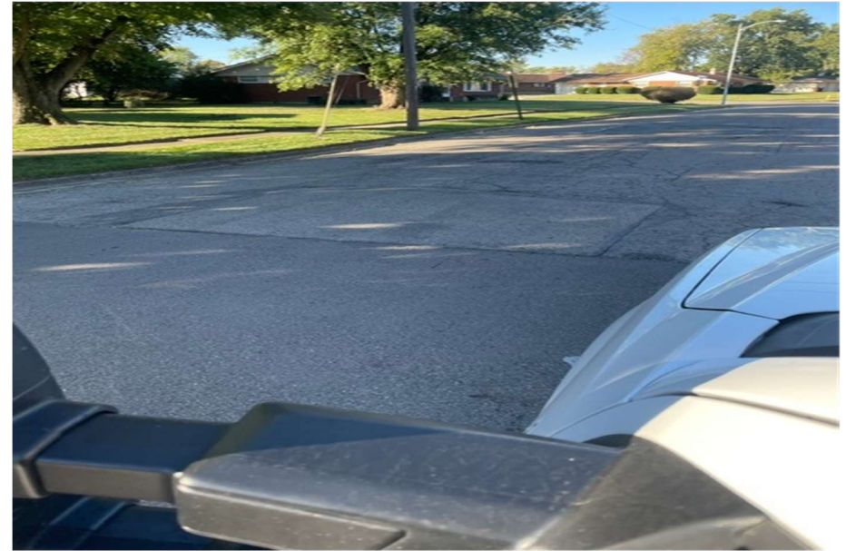
717-720 MacMillan Drive (2 Water Main Breaks)
