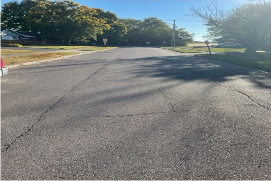
901-905 MacMillan Drive (2 Water Main Breaks)
