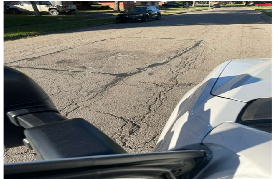
820 MacMillan Drive (1 Water Main Break)
