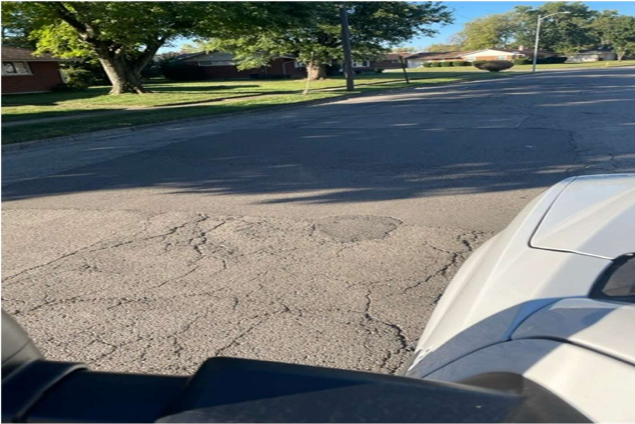
712 MacMillan Drive (3 Water Main Breaks)
