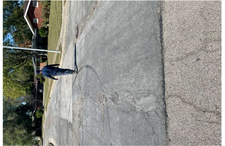
Eppington Drive and Mineola Court (2 Water Main Breaks)
