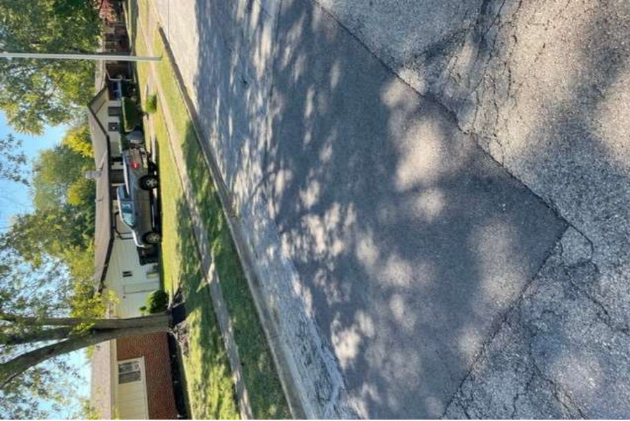
821 N. Eppington Drive (1 Water Main Break 1)
