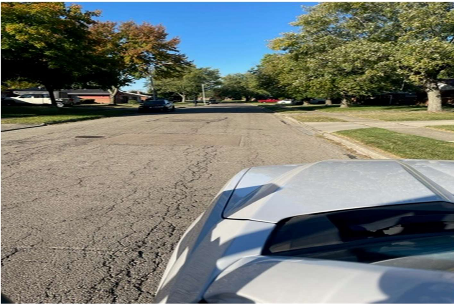
824 MacMillan Drive (1 Water Main Break)
