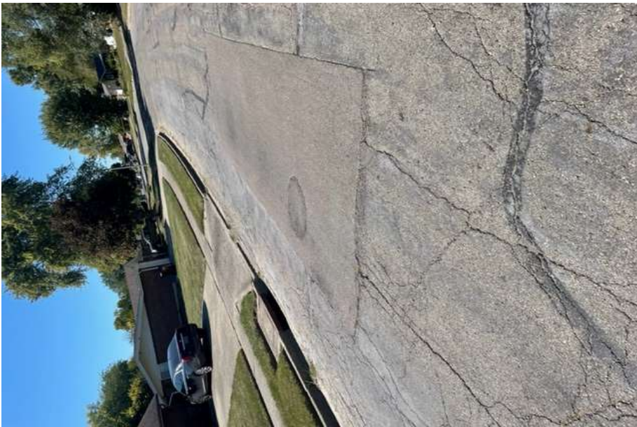
825 N. Eppington Drive (1 Water Main Break)
