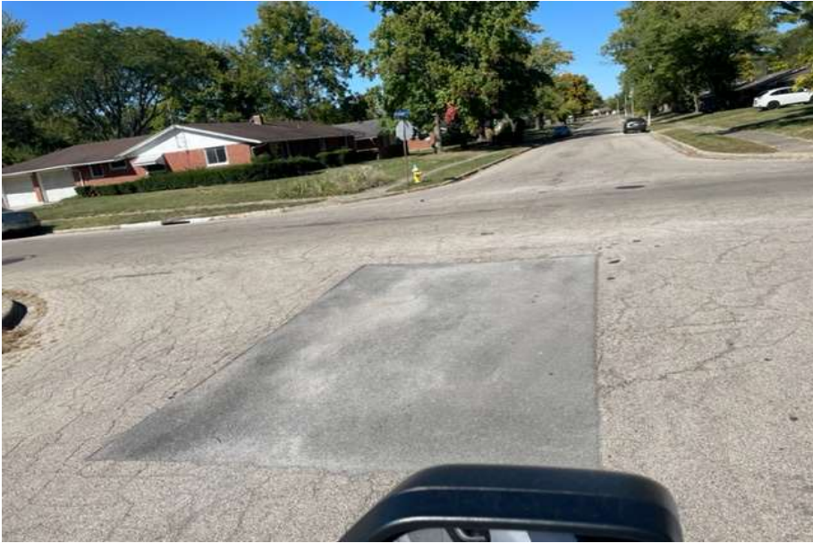
217 E. Eppington Drive (2 Water Main Breaks)
