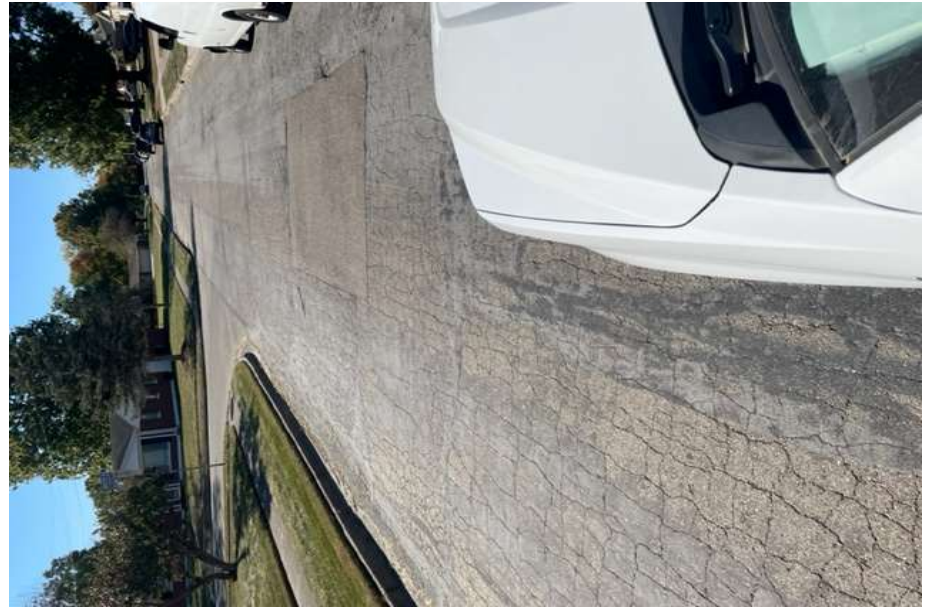
509 N. Eppington Drive (1 Water Main Break)
