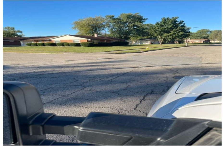
627 MacMillan Drive (1 Water Main Break)
