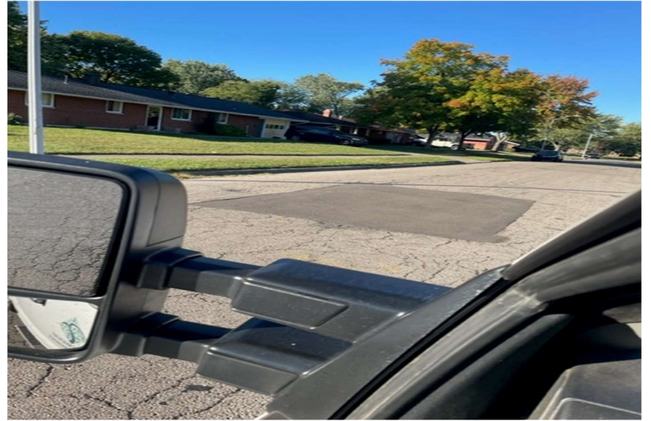
829 MacMillan Drive (1 Water Main Break)
