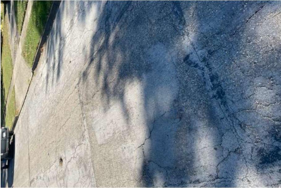
800 N. Eppington Drive (1 Water Main Break 1)
