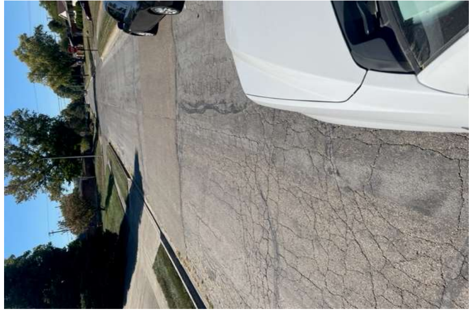
601 N. Eppington Drive (1 Water Main Break)
