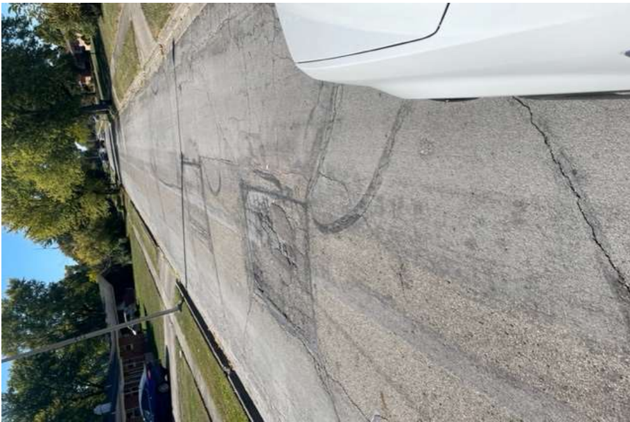
712 N. Eppington Drive (2 Water Main Breaks)
