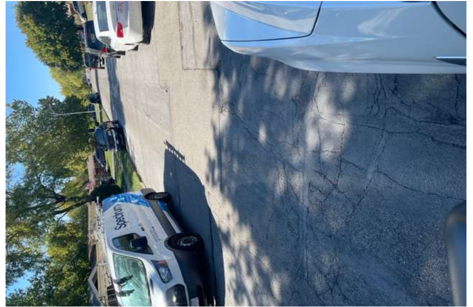
801 N. Eppington Drive (1 Water Main Break)
