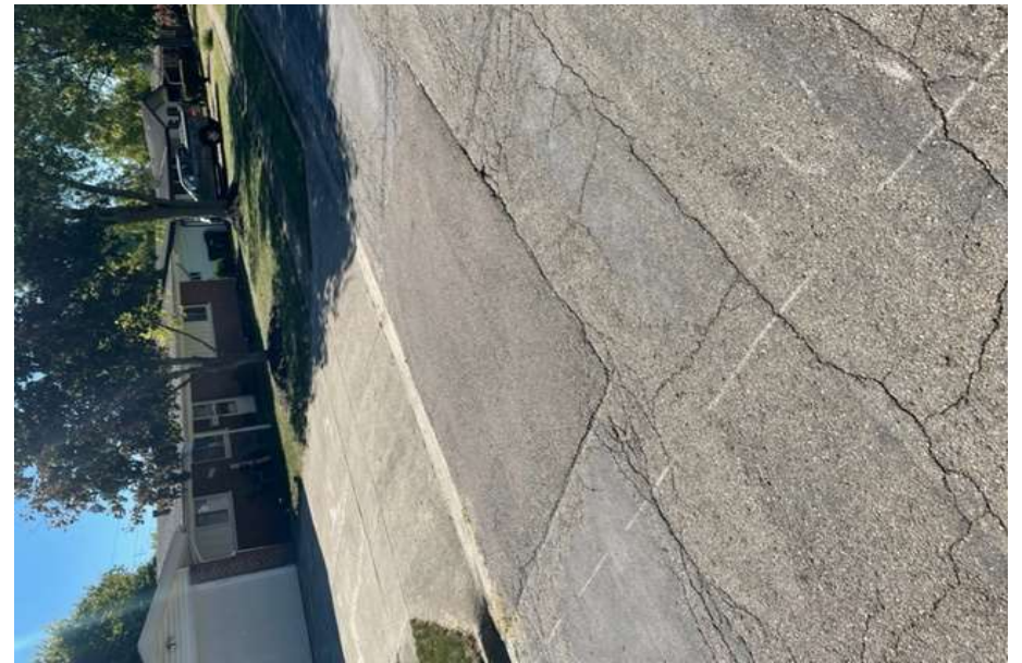
820 N. Eppington Drive (1 Water Main Break)
