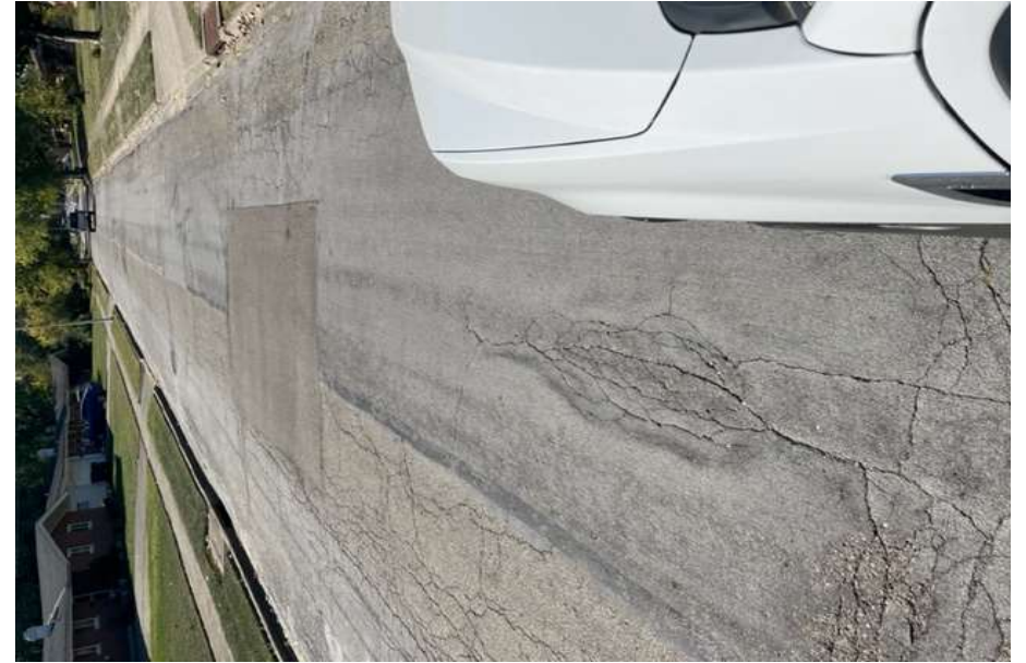
716 N. Eppington Drive (1 Water Main Break)
