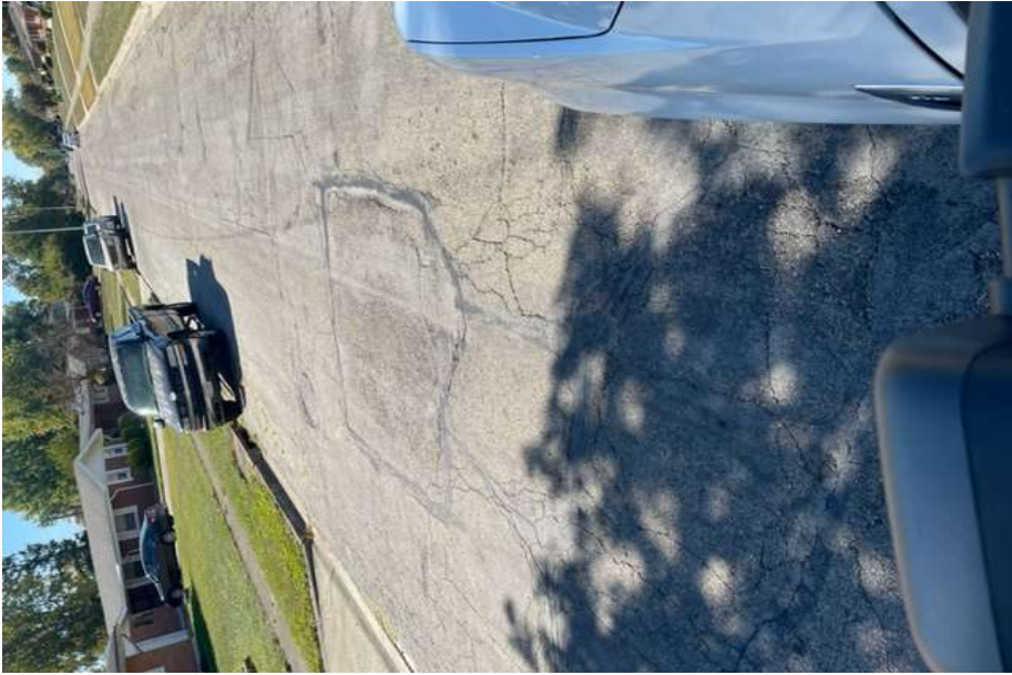
616 N. Eppington Drive (1 Water Main Break 1)
