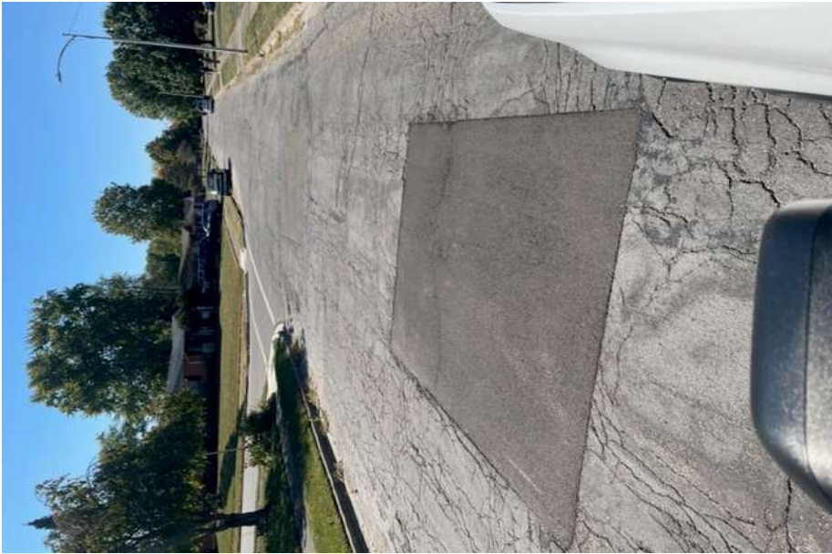
520 N. Eppington Drive (2 Water Main Breaks)
