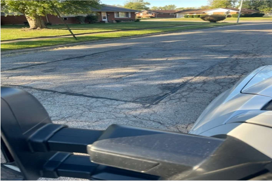
701 MacMillan Drive (1 Water Main Break)
