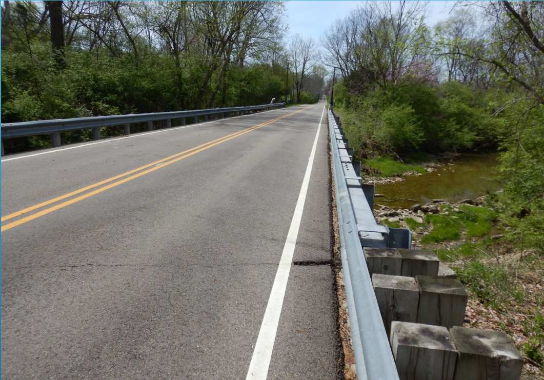
On the roadway looking west along the north side of Shank Road the bridge.
